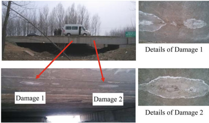
Fig. 17 The damage inspection of Yu Lin Bridge
