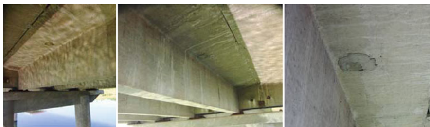
Fig. 16 The damages on the Chao He Bridge
