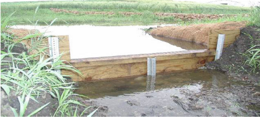
Fig. 8.4 Rectangular weir at the inlet of the pond, which was later modified
