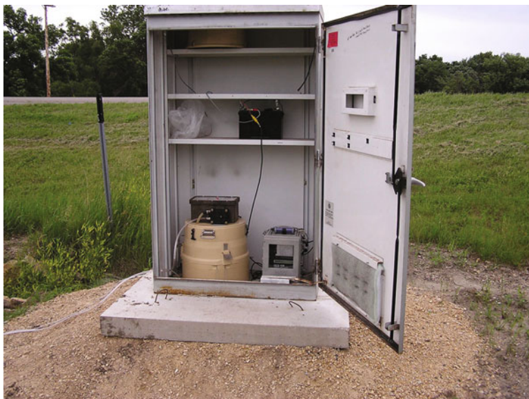
Fig. 10.5 Protective cabinet housing automatic sampling equipment
