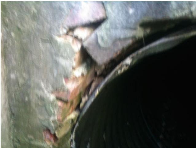
Fig. 5.5 A cracked brick and mortar outlet (©Stormwater Maintenance, LLC, www.SWMaintenance.com , reprinted with permission)
