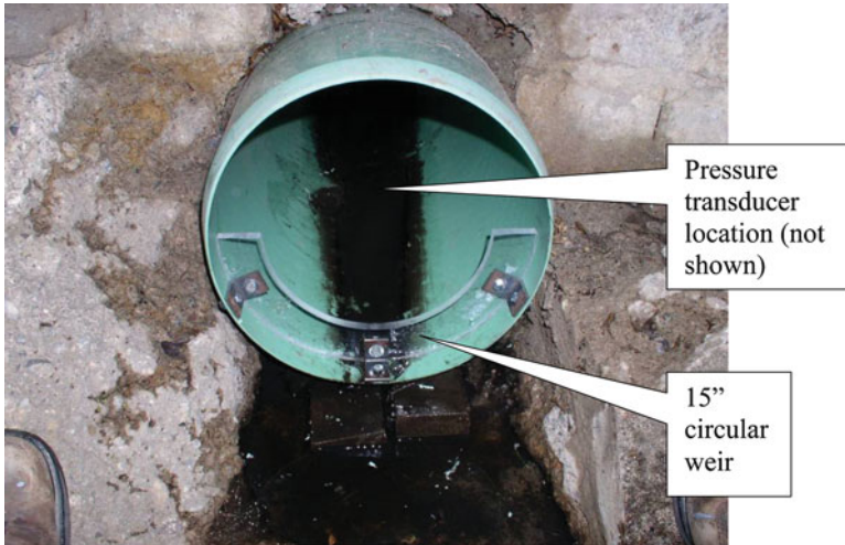
Fig. 7.3 Precalibrated 15-in. (38-cm) circular weir installed downstream of the device. Pressure transducer and transducer anchoring are not shown. This weir location provided free outfall conditions at all flow rates due to the PVC pipe's favorable elevation vs. the existing 36-in. RCP it discharged into
