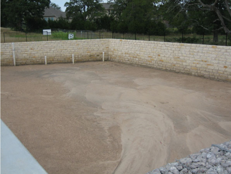
Fig. 4.7 Austin sand filter from Austin, TX
