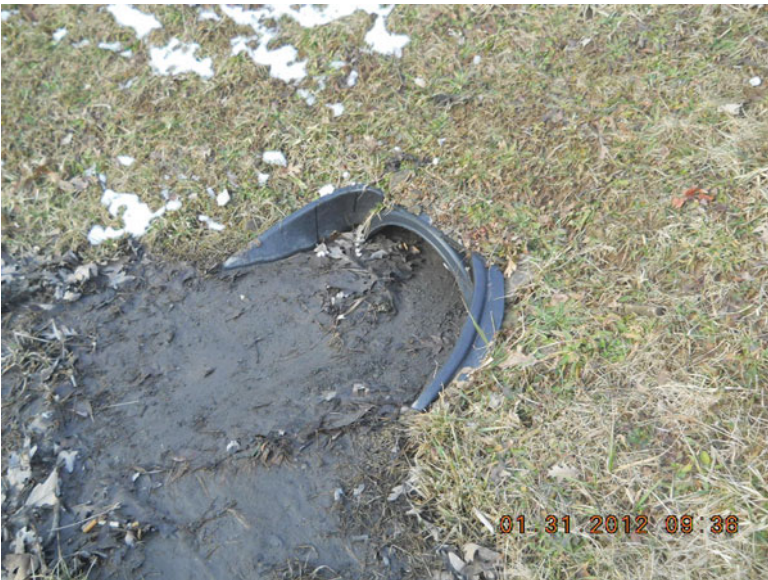
Fig. 5.9 An outlet to a stormwater treatment practice that is clogged with excessive sediment deposition (©Stormwater Maintenance, LLC, www.SWMaintenance.com , reprinted with permission)
