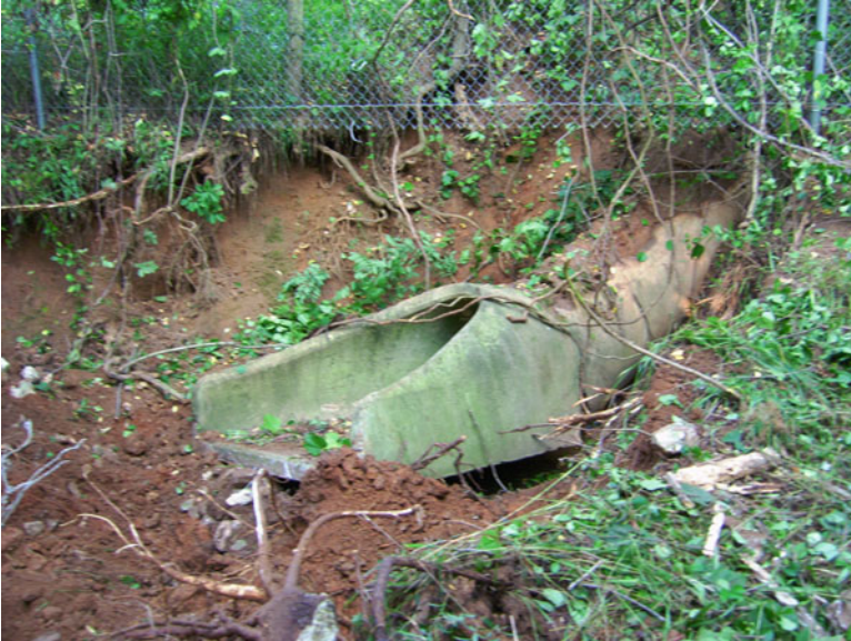
Fig. 5.6 A misaligned flared-end concrete pipe section that is also subject to excessive erosion (©Stormwater Maintenance, LLC, www.SWMaintenance.com , reprinted with permission)
