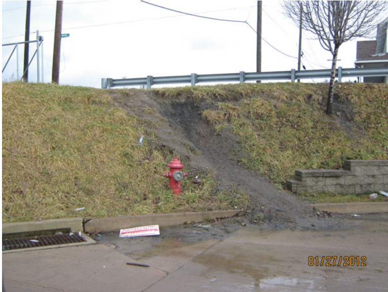
Fig. 5.11 Side slope erosion at an unintended flow entrance. Note also the tree growing on a constructed slope, which may cause soil failure (©Stormwater Maintenance, LLC, www.SWMaintenance.com , reprinted with permission)
