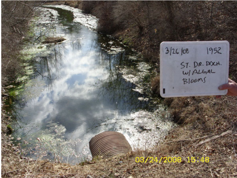
Fig. 5.18 Algal bloom in a drainage swale with standing water (©Stormwater Maintenance, LLC, www.SWMaintenance.com , reprinted with permission)
