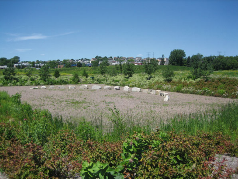
Fig. 4.9 Photo of a Minnesota Filter in Maplewood, MN. The large rocks serve aesthetic purposes
