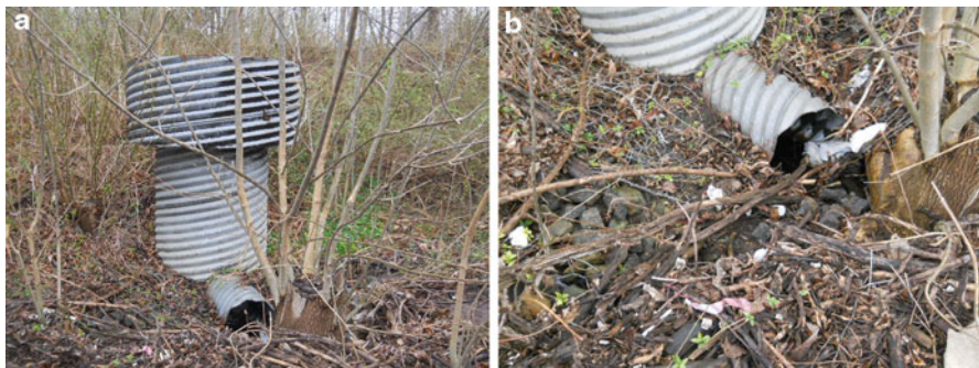
Fig. 5.3 (a) A staged outlet structure overcome with excessive vegetation (©Stormwater Maintenance, LLC, www.SWMaintenance.com , Reprinted with permission). (b) Close-up of the low-flow outlet showing that the outlet has been partially blocked by vegetation that has also trapped litter and debris (©Stormwater Maintenance, LLC, www.SWMaintenance.com , reprinted with permission)
