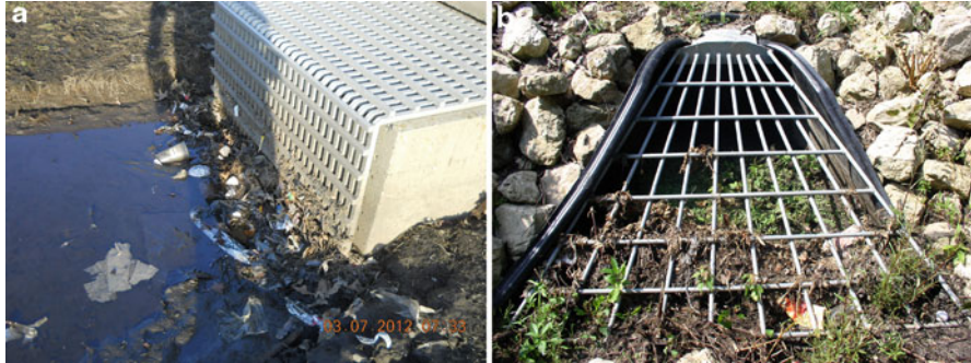
Fig. 5.2 (a) A clogged outlet structure that has caused standing water to develop within the practice (©Stormwater Maintenance, LLC, www.SWMaintenance.com , reprinted with permission). (b) Inlet structure clogged with debris
