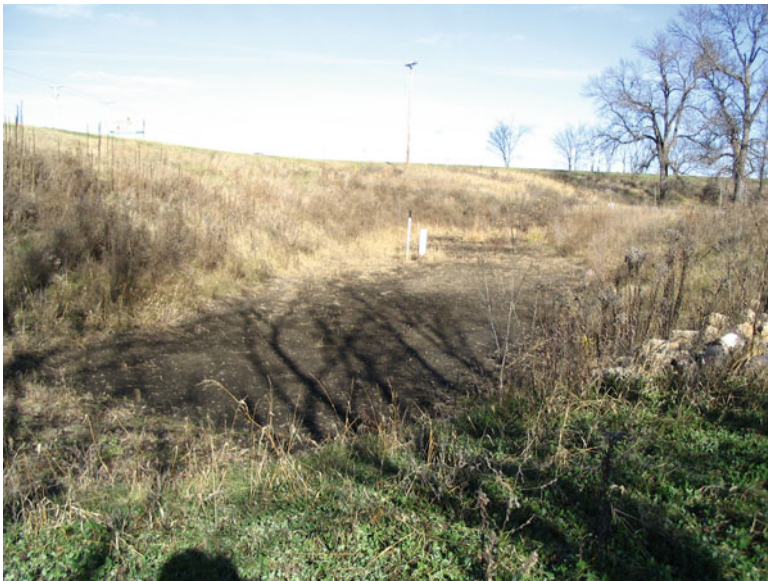
Fig. 5.17 Infiltration basin without plants indicates that the basin is not sufficiently infiltrating and standing water has prevented plants from growing
