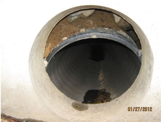
Fig. 5.4 A misaligned outlet structure pipe (©Stormwater Maintenance, LLC, www.SWMaintenance.com , reprinted with permission)
