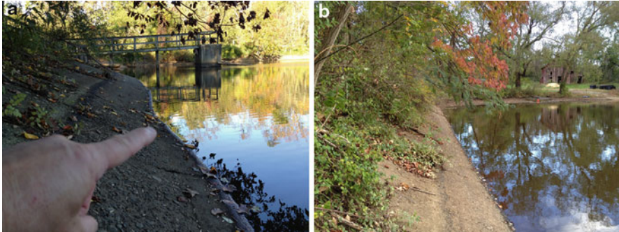
Fig. 5.12 (a) A bank of a stormwater pond that has subsided (©Stormwater Maintenance, LLC, www.SWMaintenance.com , Reprinted with permission). (b) A bank of a stormwater pond that has no evidence of soil instability or erosion (©Stormwater Maintenance, LLC, www.SWMaintenance.com , reprinted with permission)
