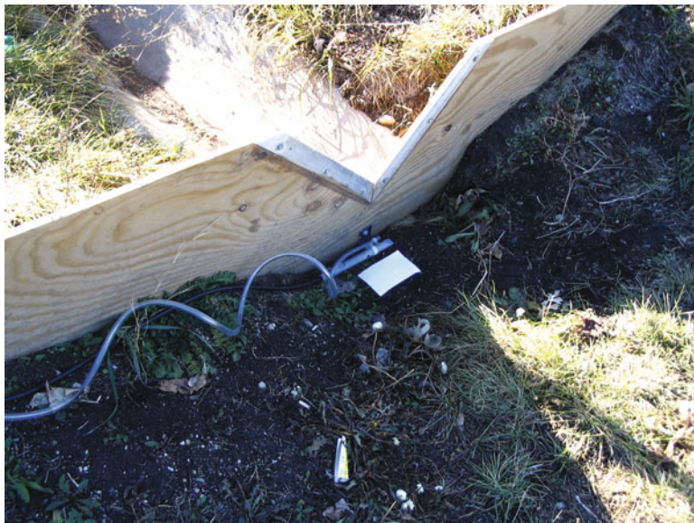
Fig. 10.4 Pressure probe for flow measurement and sampling tube for pneumatic sample collection placed at a weir to measure stormwater inflow
