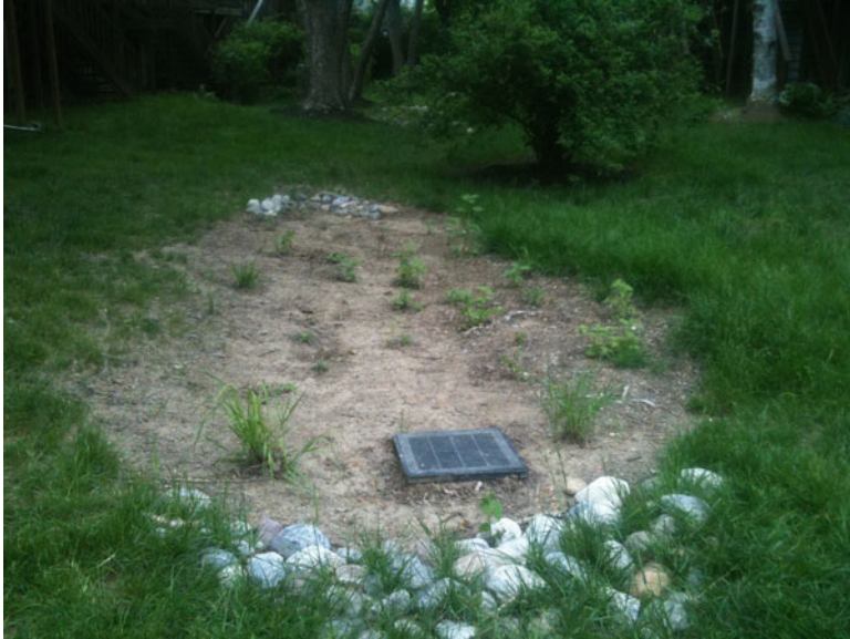
Fig. 5.10 Bare soil that indicates excessive periods of inundation with water (©Stormwater Maintenance, LLC, www.SWMaintenance.com , reprinted with permission)
