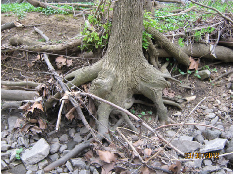
Fig. 5.7 A channel that exhibits signs of erosion through bare soil and exposed tree roots (©Stormwater Maintenance, LLC, www.SWMaintenance.com , reprinted with permission)
