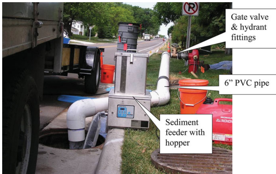
Fig. 7.4 Piping system from hydrant to influent injection point and stainless steel sediment feeder
