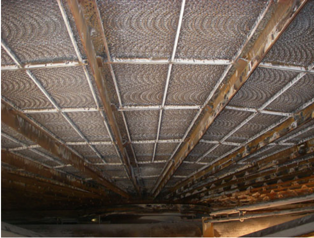
Fig. 9.11 View from underneath the rotor (Courtesy of Millmerran Operating Company, Australia)
