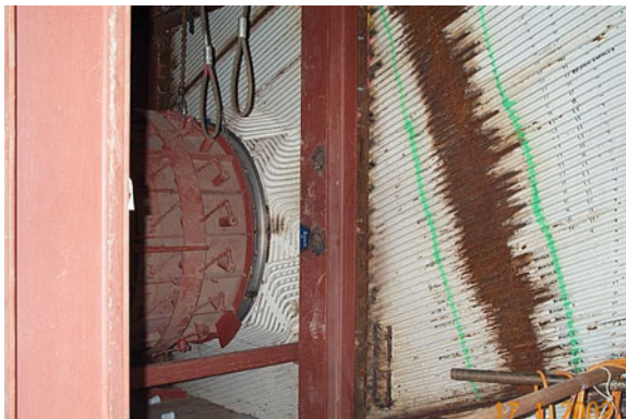
Fig. 11.11 A wall-mounted burner with surrounding wall tubes (Courtesy of Millmerran Operating Company, Australia)
