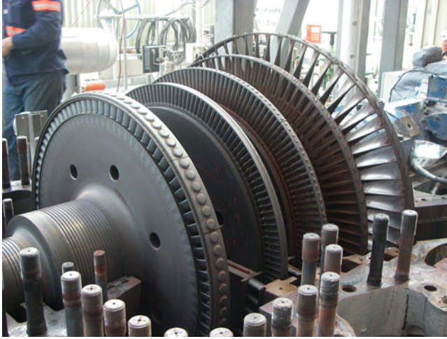
Fig. 14.1 A boiler feedpump turbine, open for inspection (courtesy of Millmerran Operating Company, Australia)
