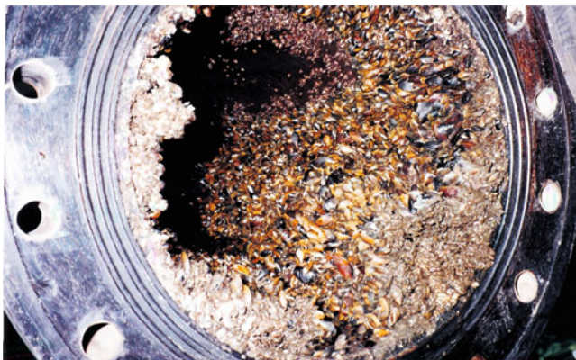
Fig. 1.4 Blockage of the seawater pipe at a power station by biofouling growth
