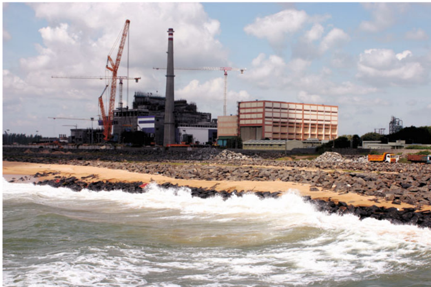
Fig. 1.5 A nuclear power plant being constructed close to the seacoast. Cooling water availability is a major criterion that influences power plant siting
