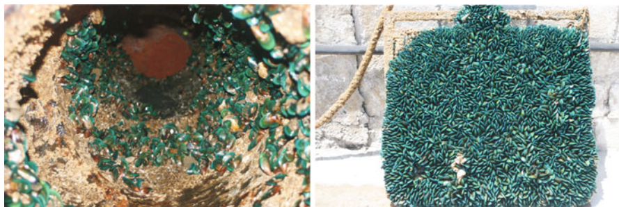
Fig. 1.3 Fouling by green mussels ( Perna viridis ) inside a seawater intake pipe (left) and on test coupons placed in the sea (right)
