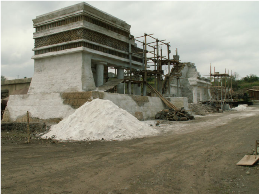
Fig. 8.22 Construction of a Postclassic period structure with a large mound of lime in the foreground (Photo: R.D. Hansen)
