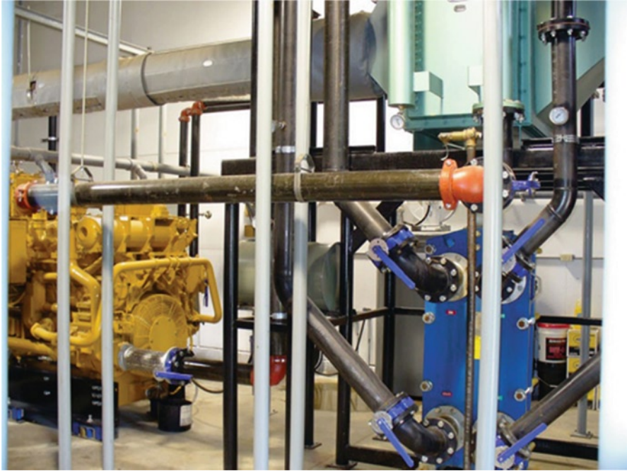
Fig. 2.9 A heat exchanger working with a biogas-fed engine-generator set to utilize heat for space and water heating (photo courtesy: AgSTAR)
