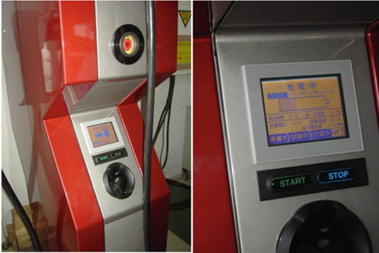
Fig. 9.40 CHAdeMO charger at TEPCO, Yokohama
