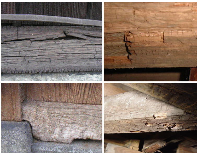
Fig. 14.50 Wood decay in final stages
