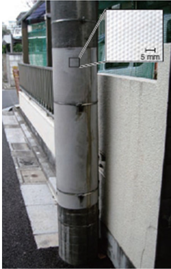
Fig. 14.12 Bill-posting prevention sheet on a concrete pole
