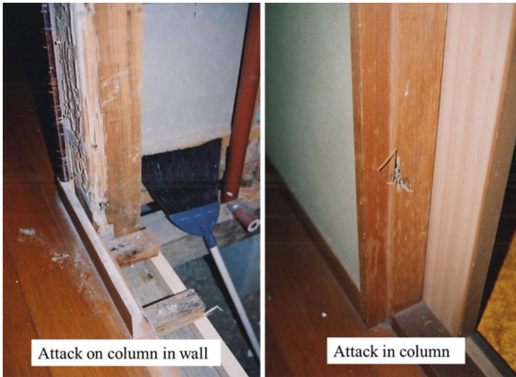
Fig. 14.54 Termite attacks developing in wooden wall
