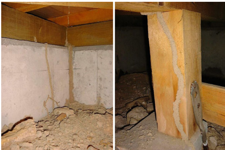
Fig. 14.52 Termite galleries developed on wood under floor level
