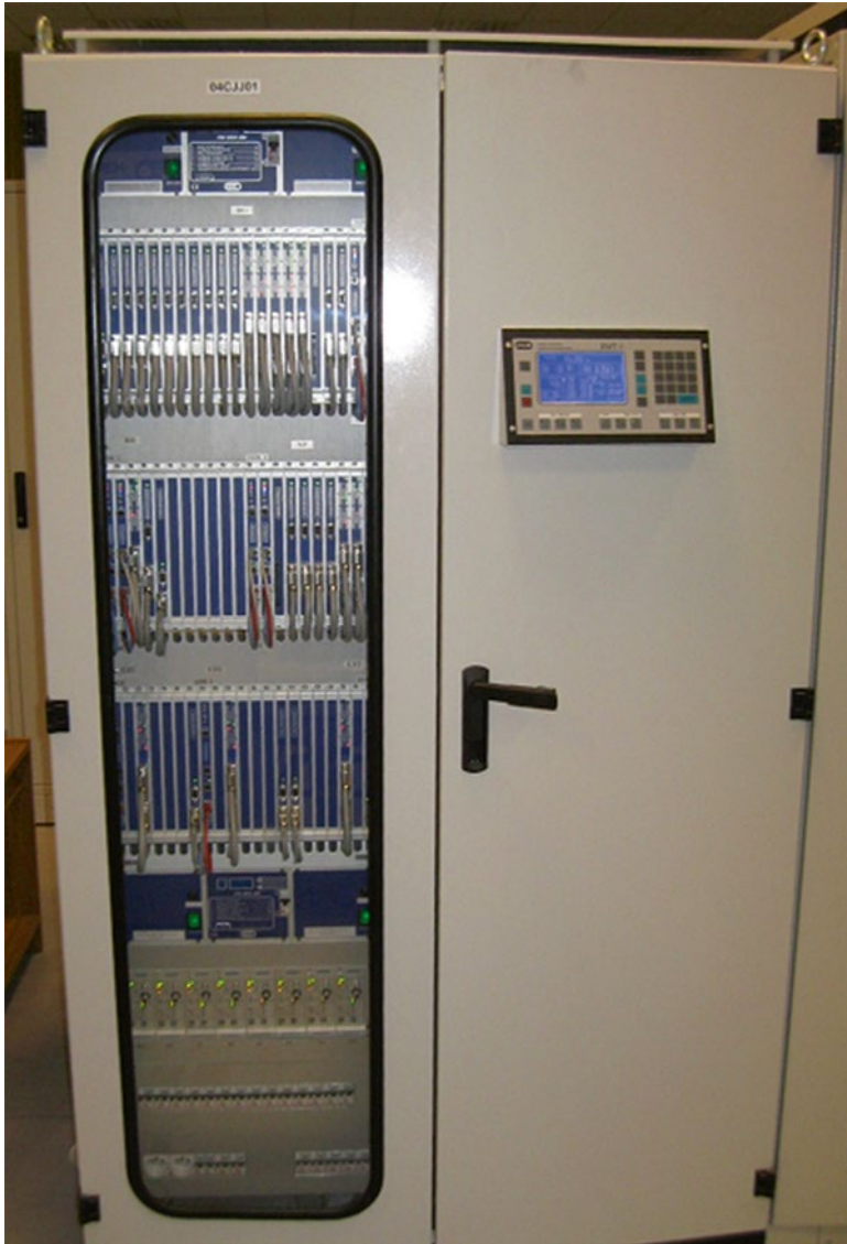
Fig. 8.19 Front panel of an automation cabinet
