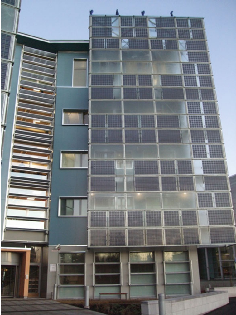
Fig. 12 PV installation on the double facade to south serving also as an effective solar shading
