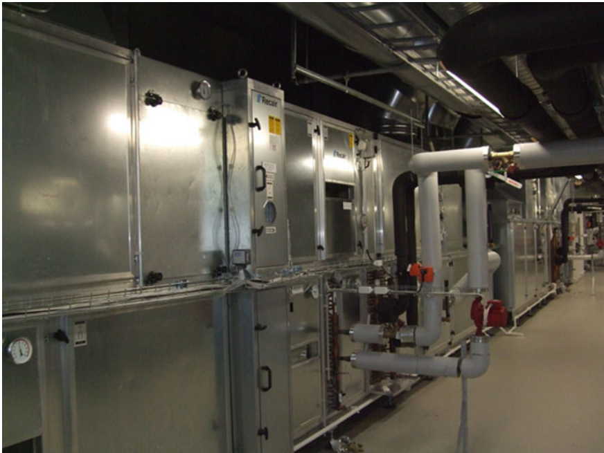
Fig. 14 Large air handling units and ductworks have been used to achieve as low-specific fan power as 1.4–1.6 kW/(m 3 /s) for offices and similar spaces and 1.8 kW/(m 3 /s) for VAV air handling unit serving meeting rooms
