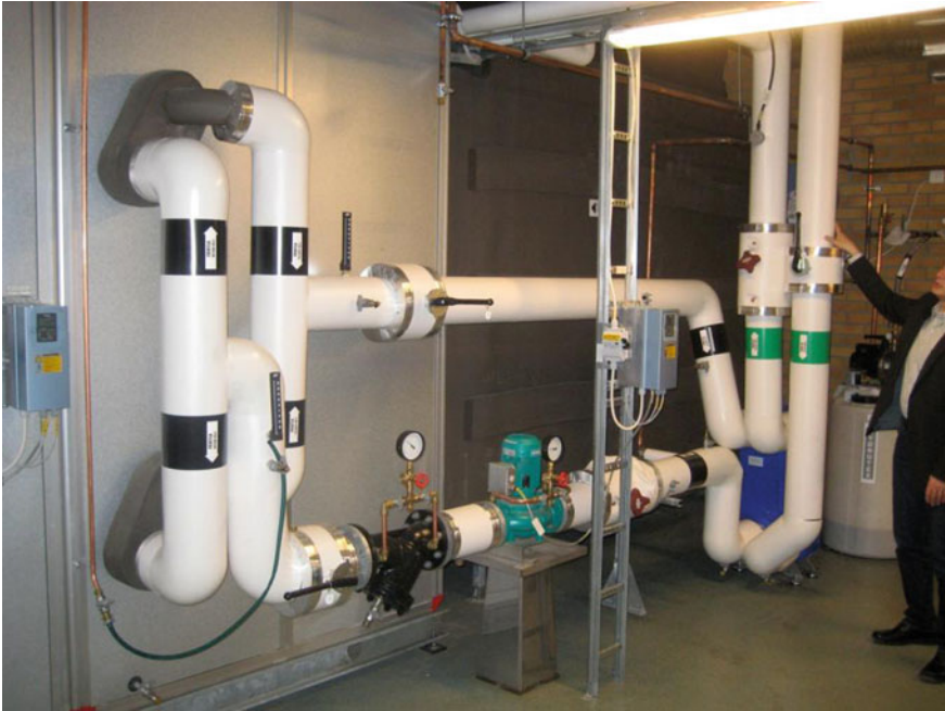
Fig. 27 Free cooling coil in AHU cools the chilled water system and preheats the supply air
