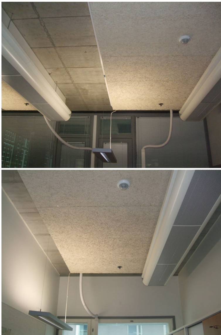
Fig. 15 Active chilled beams and lighting fittings in offices
