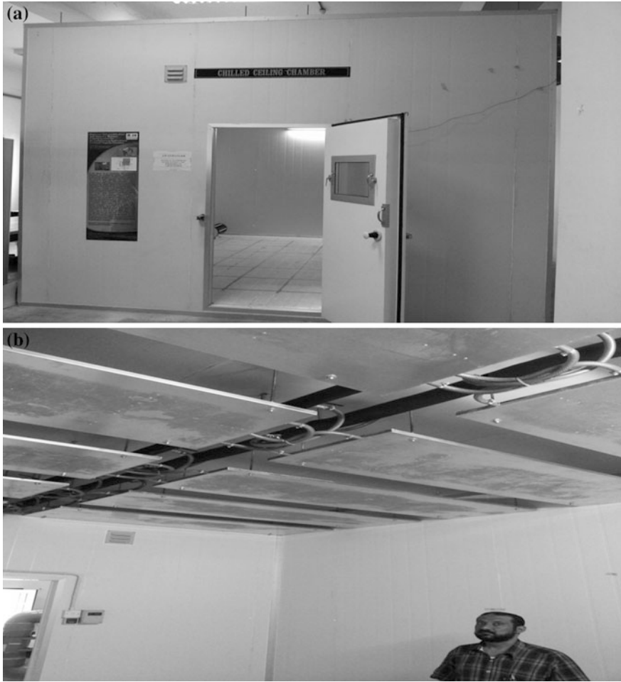
Fig. 3 Environmental chamber with installing chilled ceiling panels
