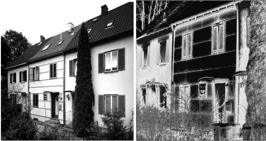
Fig. 14 View of a refurbished terraced house. Left picture photography and right picture thermal image. The dark colours of the thermal image correspond to low surface temperatures and therefore are an indicator for an excellent thermal insulation
