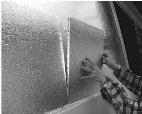
Fig. 11 Installation of the VIP on the top of the vapour barrier. In the edge regions, triangular-shaped VIPs were used
