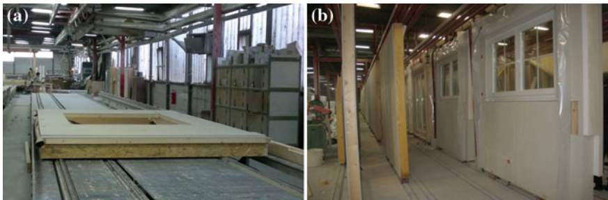
Fig. 3.35 The walls with openings are constructed in horizontal position (a) and then put in vertical position (b)
