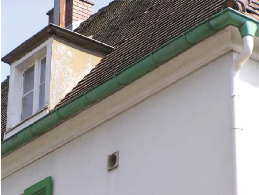
Fig. 4.8 Most German houses do not have overhangs on all sides wide enough to accommodate 12 cm of extra insulation as required by the EnEV
