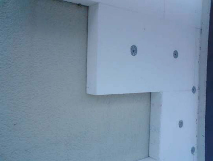
Fig. 4.3 Wall insulation is usually glued and screwed to the outside surfaces of the walls and covered with a render
