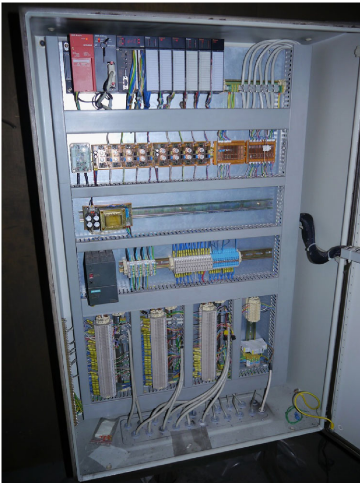
Fig. 7.21 Implementation of the control cabinet
