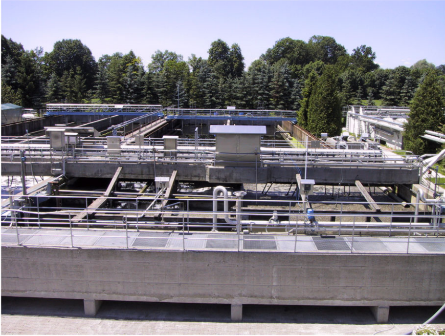
Fig. 5.5 Photo of the pilot plant
