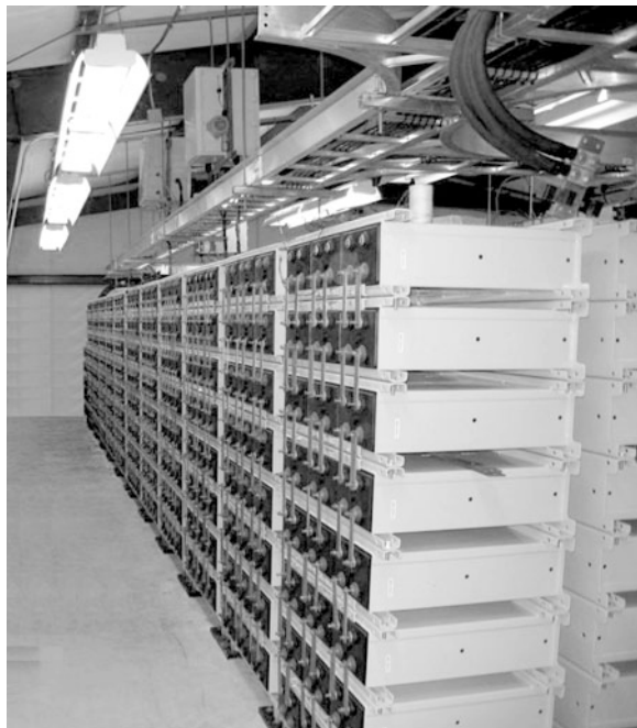
Fig. 9.3 A portion of the BESS at Metlakatla, Alaska that uses GNB ABSOLYTE IIP 100A75 modules. Seen is one bank of a back-to-back row
