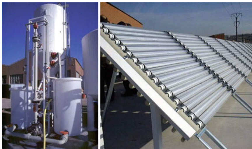
Fig. 3.4 Solar water detoxification demonstration plant installed at Hidrocen factory (Madrid, Spain). Left \text{TiO}_2 separation system. Right CPC photoreactor field (Malato et al. 2009). Copyright Elsevier. Reproduced with permission
