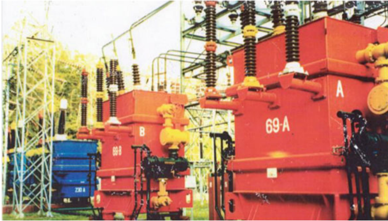
Fig. 1.8 Substation voltage transformers
