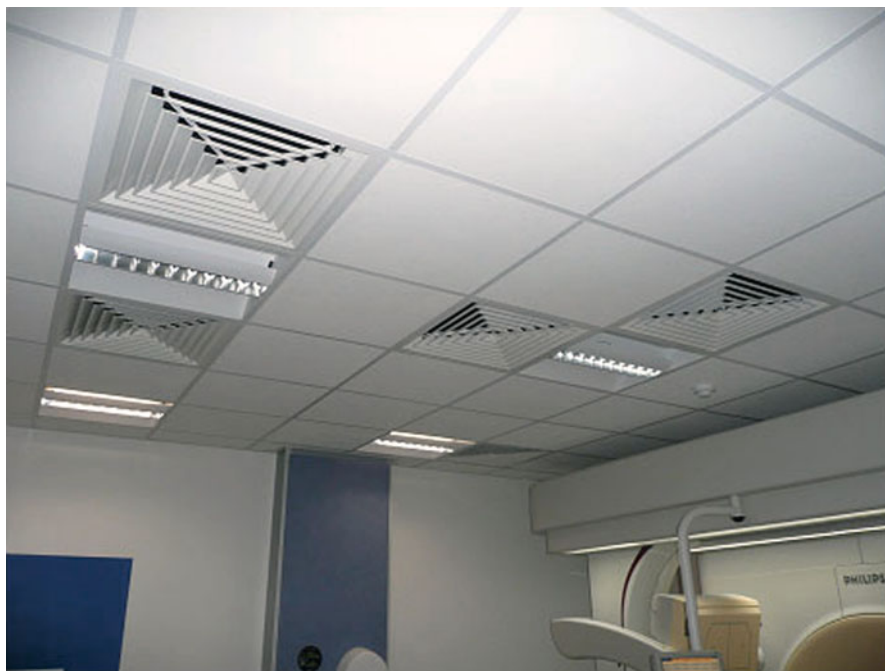
Fig. 7.5 Air diffusers (grilles in the ceiling) ensuring uniform air temperature
