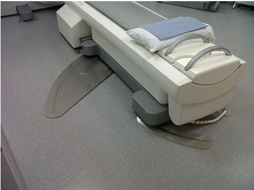
Fig. 6.11 Installation of floor plates to preserve the alignment of the patient imaging pallet to the gantry
