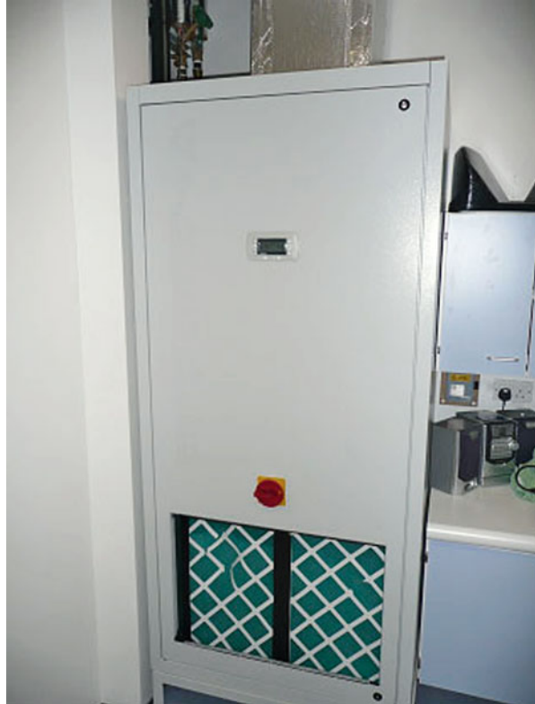
Fig. 7.4 High-capacity climate-control plant installed in a scanning room
