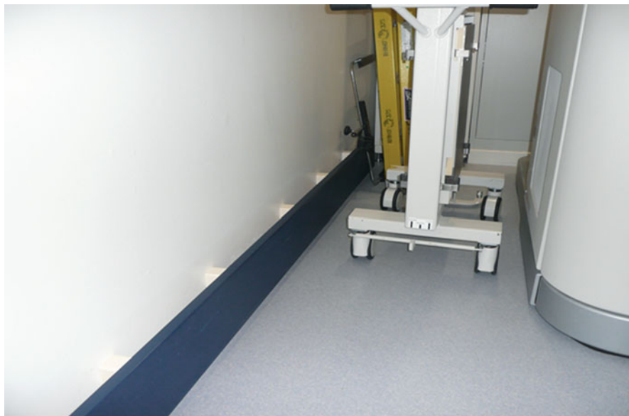
Fig. 7.3 This figure demonstrates the use of plastic kickboards which serve to protect the wall
