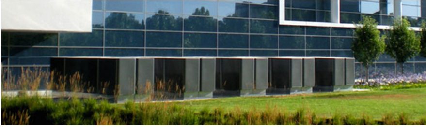
Fig. 10 Five 100 kW sized SOFC systems (Bloom Boxes) installed at eBay Headquarters
