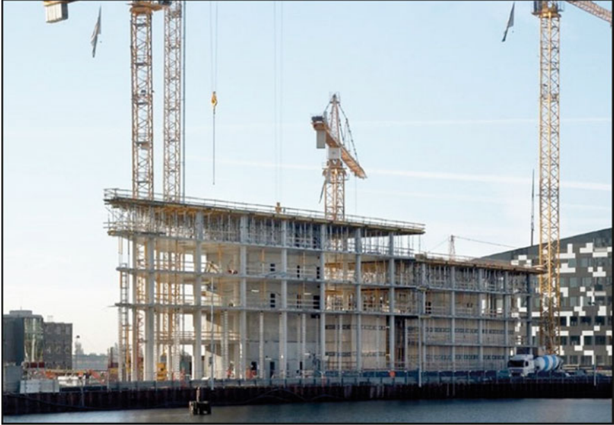
Fig. 4.9 The superstructure rises. Note how the columns are placed directly beneath each other in order to accommodate load bearing. Also, note the formwork supporting the casting of the upper decks as well as the cement truck used in the process
