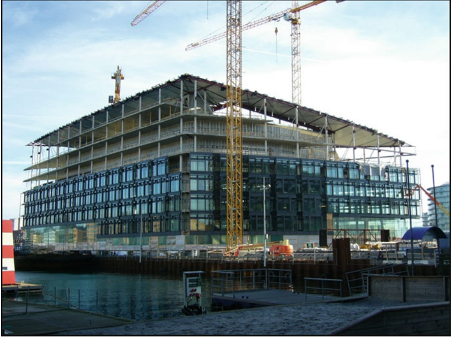
Fig. 4.11 The domicile half covered in façade panels and with some sections of the roof set in place
