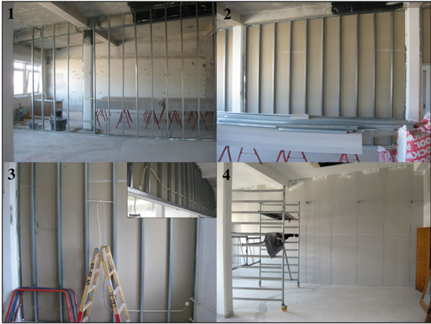
Fig. 7.8 Interior wall in-the-making. The first and second frame shows the result of the carpenter's initial efforts. The third frame, including insert , shows the work of the electrician in progress. Finally, the fourth frame depicts the closed wall ready for painting
