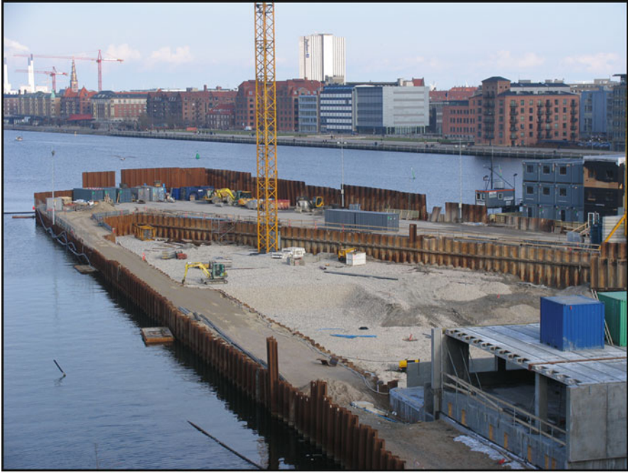
Fig. 4.8 The construction site of one of the buildings studied, i.e. the domicile (Image is courtesy of PLH Architects A/S. Reproduced with permission)
