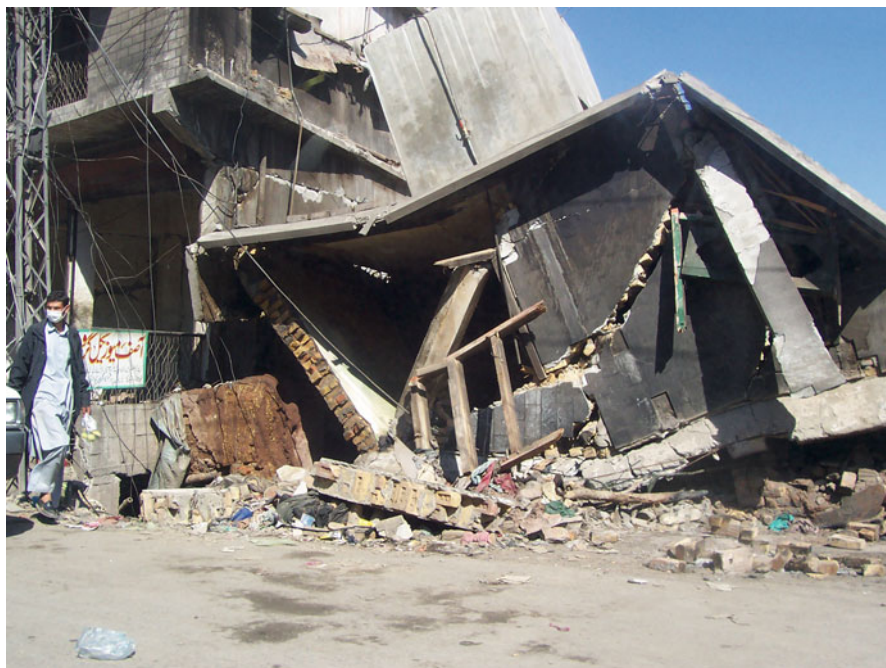
Fig. 7.1 Earthquake damage in Muzaffarabad, Pakistan, October 2005
