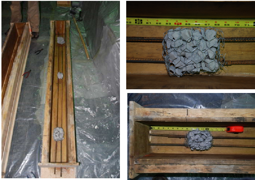
Figure 11: Rock pocket defects are intentionally located in the concrete beam.
