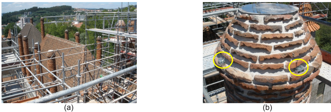
Figure 8 - Chimneys at Paço dos Duques Building. (a) Current restoration works and, (b) Sensors location.
