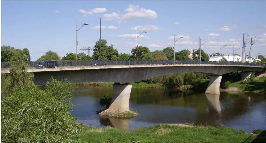
Figure 6: The Friedensbrücke-Nord in Magdeburg on which the long term monitoring system is installed
