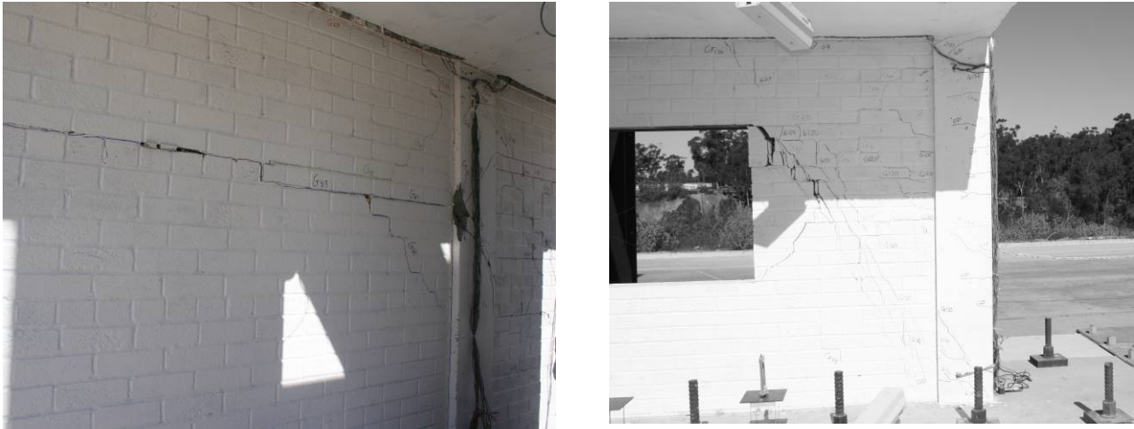
Fig. 7 Crack pattern at damage states S6 in the solid infill and the middle column (left), and the infill with opening and the east column (right)
