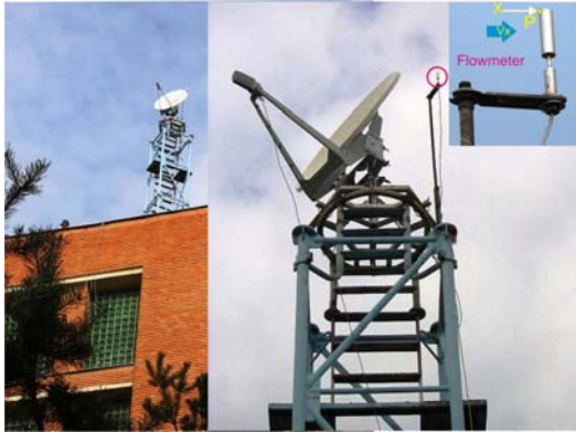
Figure 15 Illustration of the flowmeter placed on a metallic pillar on a building roof.
