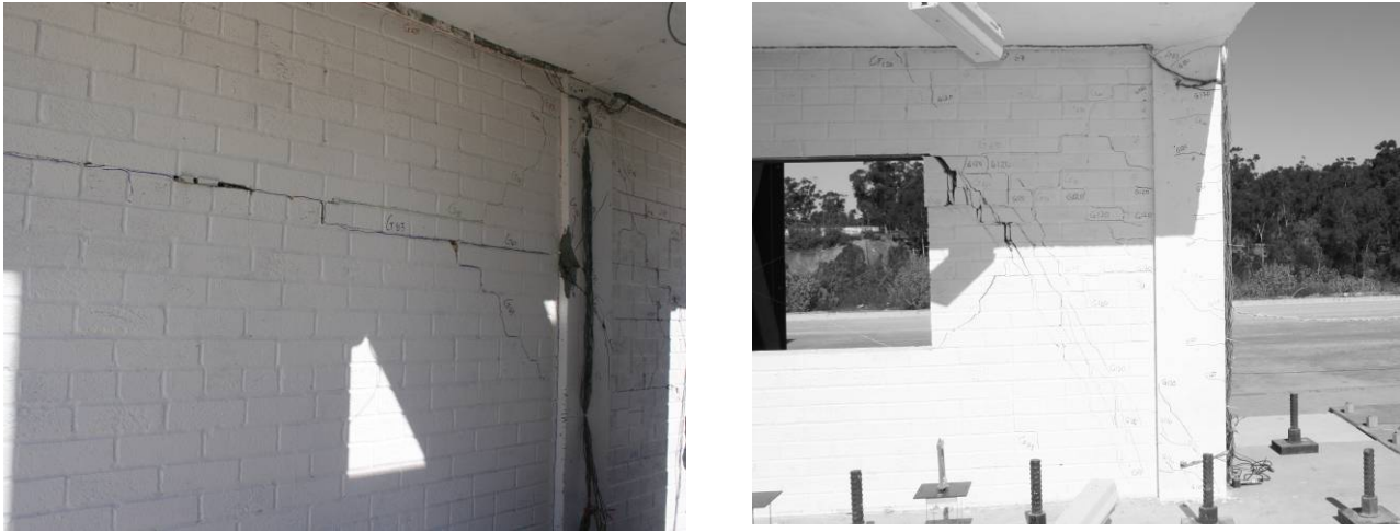
Fig. 9 Crack pattern at damage states S6 in the solid infill and the middle column (left), and the infill with opening and the east column (right)
