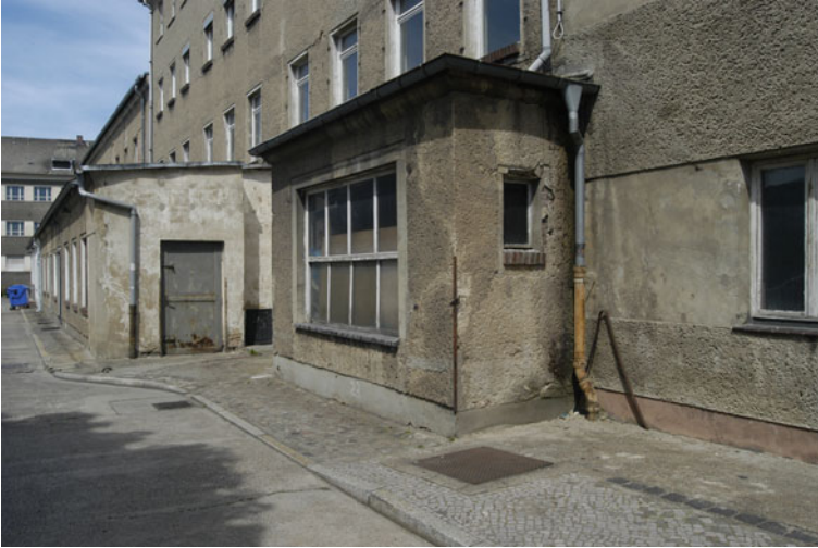
Fig. 14.13 Control office for access into Lager X, Camp X, which was mainly responsible for vehicle maintenance. Above, bars have been cut from the windows
