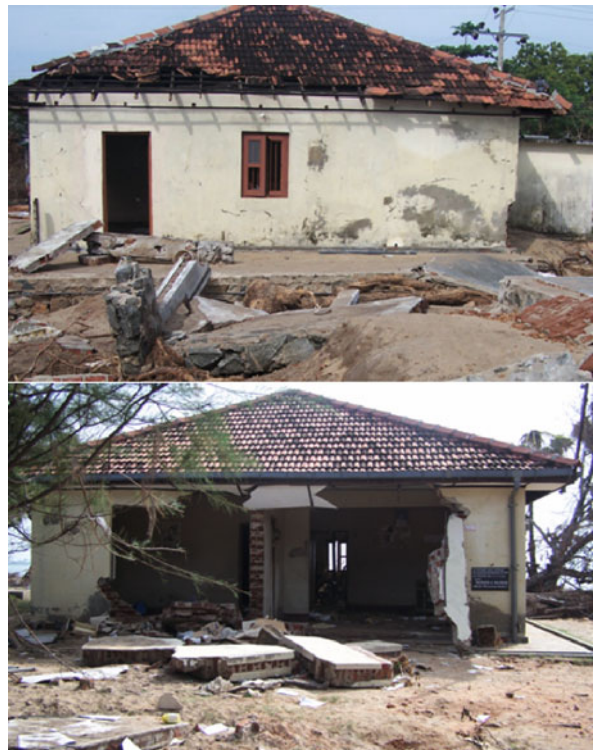
Tsunami Inundation, Modeling of, Figure 4 Example of damage to the backside of a coastal residence. These images were taken by the International Tsunami Survey Team to Sri Lanka in January 2005. The top photograph shows the front side of the structure, facing the ocean; there is damage but the main structure is intact. The lower photo shows the backside of the same building, showing the walls blown out, away from the center of the structure
