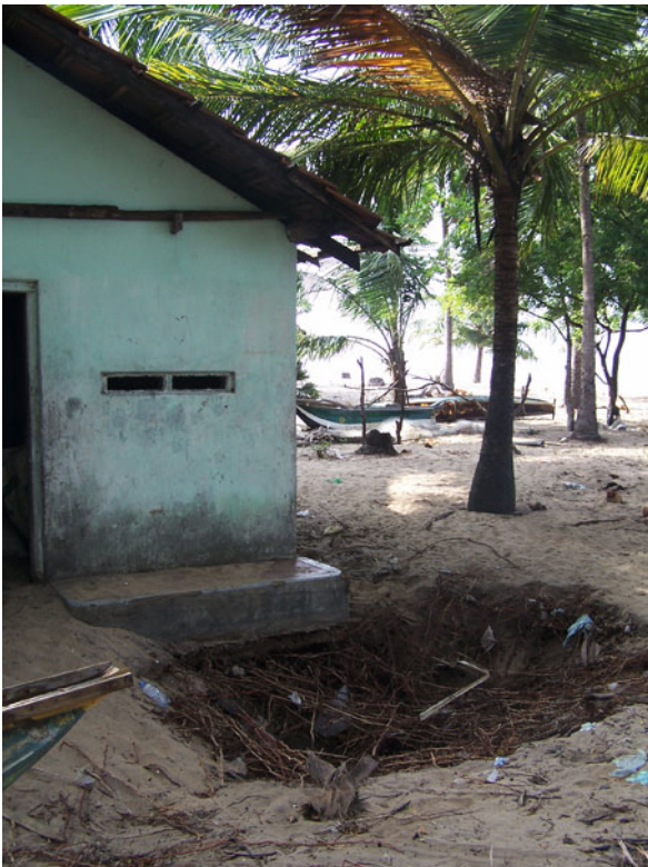
Tsunami Inundation, Modeling of, Figure 3 Example of foundation scour. This image was taken by the International Tsunami Survey Team to Sri Lanka in January 2005
