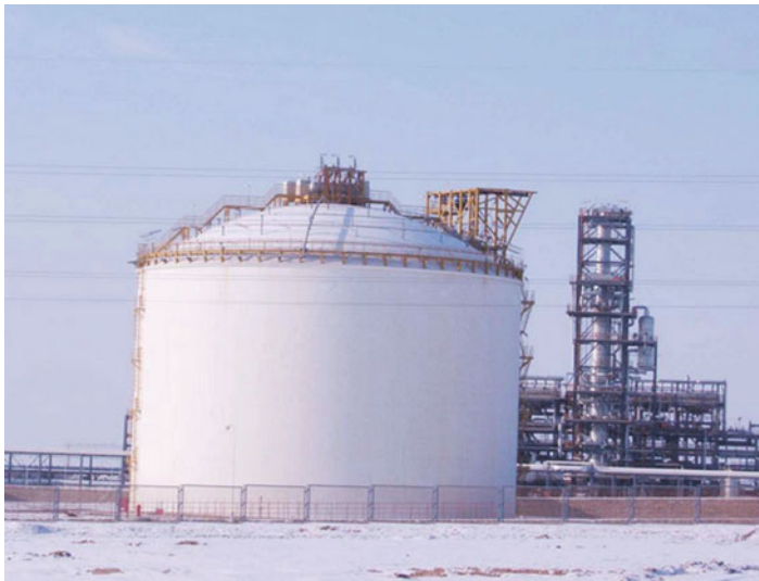
Figure 40.14. Liquid natural gas (LNG) storage tanks.
