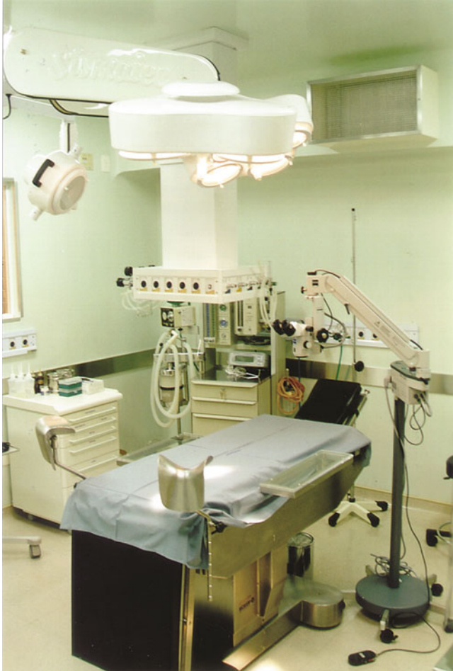
Fig. 9.16 Operating room with ceiling HEPA-filter diffuser
