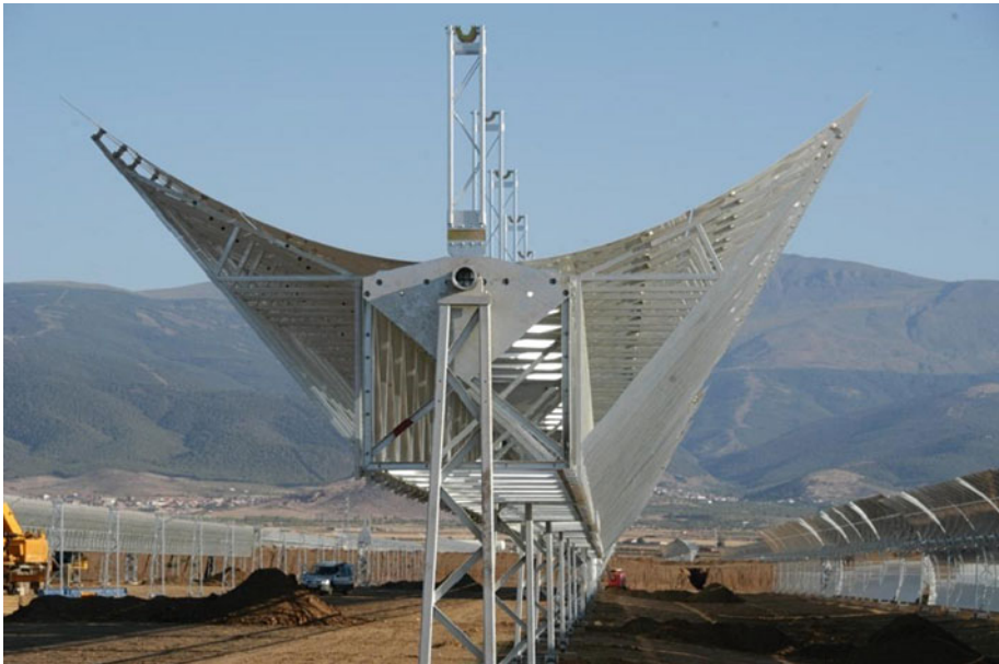
Parabolic Trough Solar Technology. Figure 12 EuroTrough support structure
