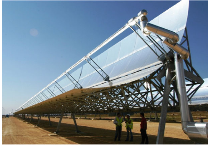
Parabolic Trough Solar Technology. Figure 5 Parabolic trough collector (EuroTrough) solar field installation
