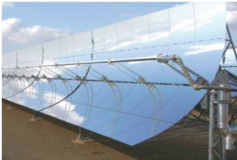
Parabolic Trough Solar Technology. Figure 4 Parabolic trough collector (EuroTrough) solar field installation
