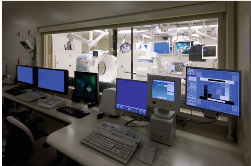
Fig. 12.6 Angiography/CT procedure room. The different displays needed in an advanced image-guided procedure room are highlighted. There needs to be PACS displays ( left ), boom-mounted displays with processed images ( right ), and patient information wall displays. Spot lights also will need to be mobile because of the mobile area of therapeutic interest (Photograph courtesy of John Bartelstone Photography)
