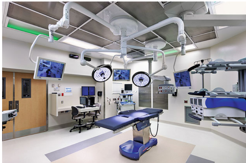
Fig. 12.4 Typical laparoscopic/MIS/general operating room. This photograph illustrates lighting requirements including ceiling lights, spot LED lights, and green light for dimmed environments. Ceiling mounts in the center of the room for laminar ceiling to floor air flow are also seen (Photograph courtesy of John Bartelstone Photography)
