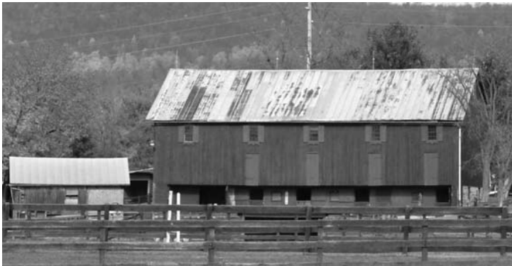
Fig. 5.8 The corrosion of a galvanized roof in the natural atmosphere. When the protective zinc coating is breached, the underlying steel eventually suffers corrosion
