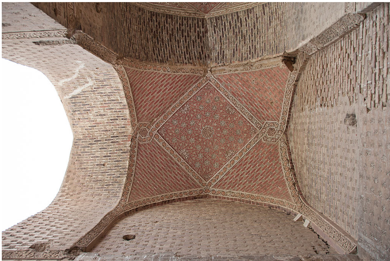
Photograph 87 An Ilkhanid vault in the mausoleum of Uljaytu in Sultaniya, Iran, with a fourfold nonsystematic median pattern comprised of 7- and 12-pointed stars (© Daniel C. Waugh)
