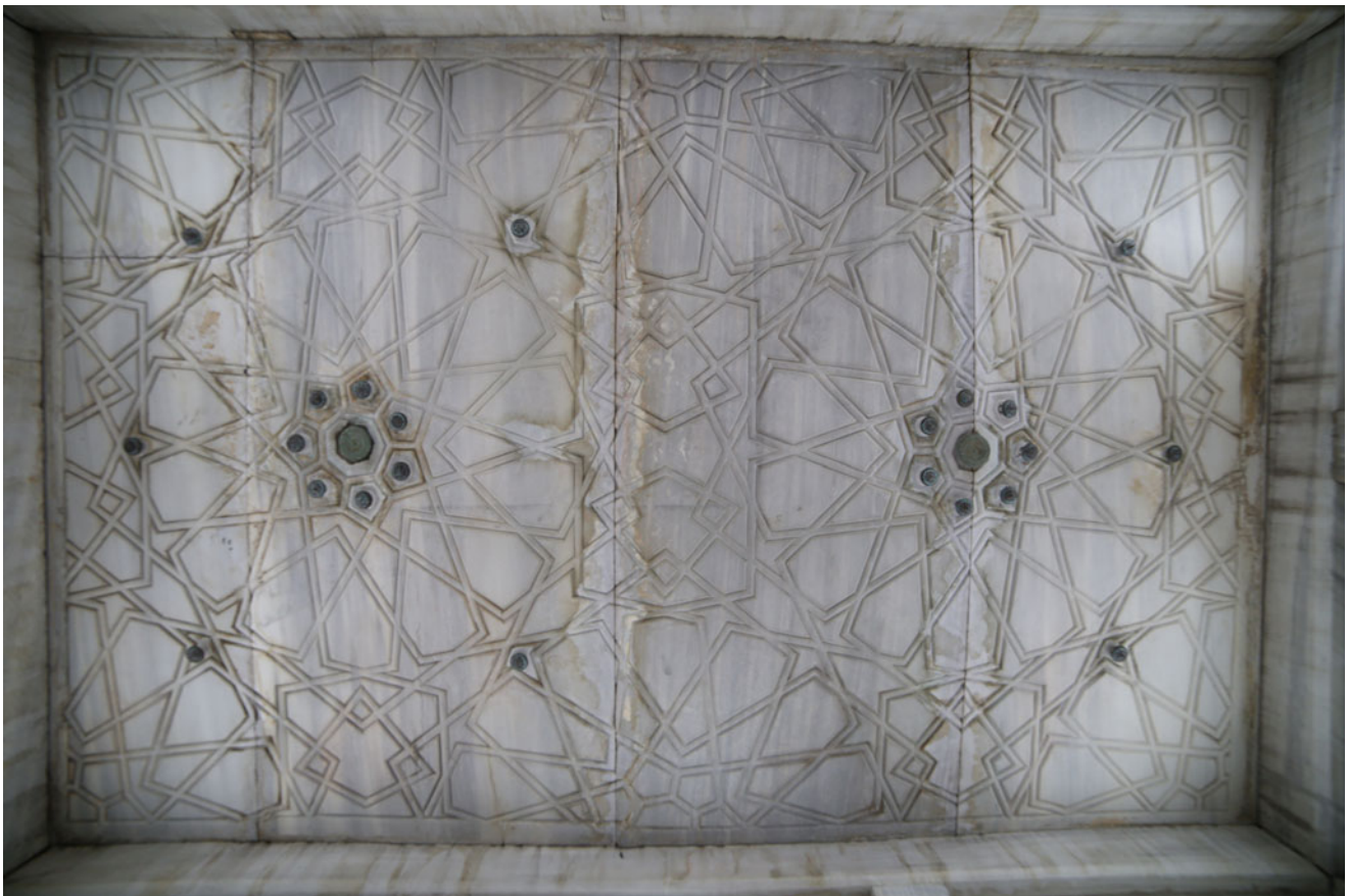
Photograph 81 An Ottoman incised stone ceiling in a water feature of the courtyard at the Suleymaniya mosque in Istanbul that employs an acute pattern created from the sevenfold system (© Serap Ekizler Sönmez)
