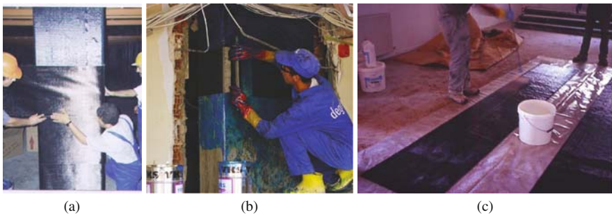
Fig. 6.3 Hand lay-up of FRPs in situ: (a), (b) dry fabric impregnated in place (courtesy A. Ilki); (c) impregnation of the fabric right before placing (See also Colour Plate 15 on page 729)
