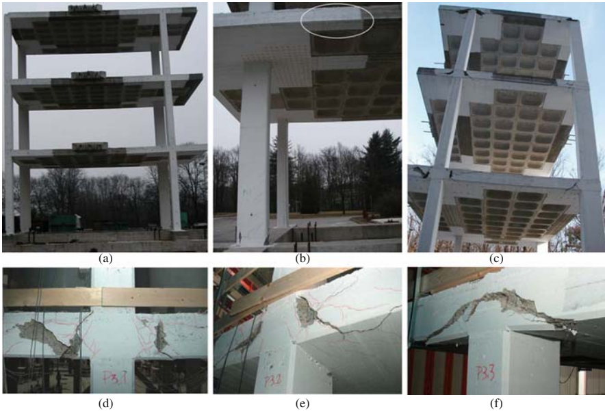
Fig. 2.17 Flat slab frame after pseudodynamic test at the ELSA laboratory of the JRC: (a) side parallel to loading; (b) hinge in slab in positive (sagging) bending and plastic hinges at column base; (c) side at right angles to loading, with slab damage around connections; (d) edge slab-column connection, 1st floor; (e) edge slab-column connection, 2nd floor; (f) edge slab-column connection, 3rd floor (pictures (d)–(f) courtesy F. Taucer, JRC). (See also Colour Plate 5 on page 719)
