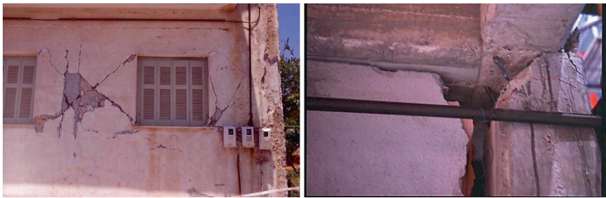
Plate 2 Examples of shear failure of weak columns interacting with strong infills. (See also Figure 2.11 on page 79)
