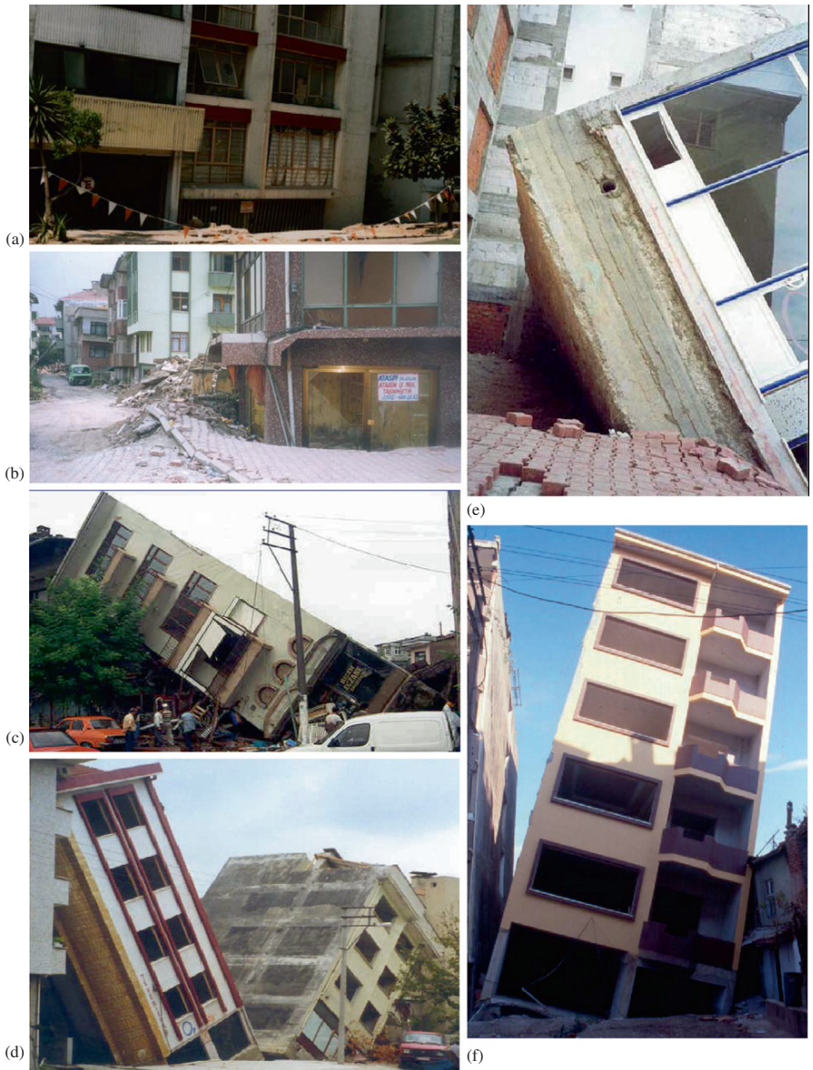
Plate 6 Bearing capacity failures at: (a) in Mexico City (1985) (b)–(f) Adapazari (TR) in the 1999 Kocaeli earthquake (courtesy G. Gazetas, NTUA). (See also Figure 2.18 on page 109)
