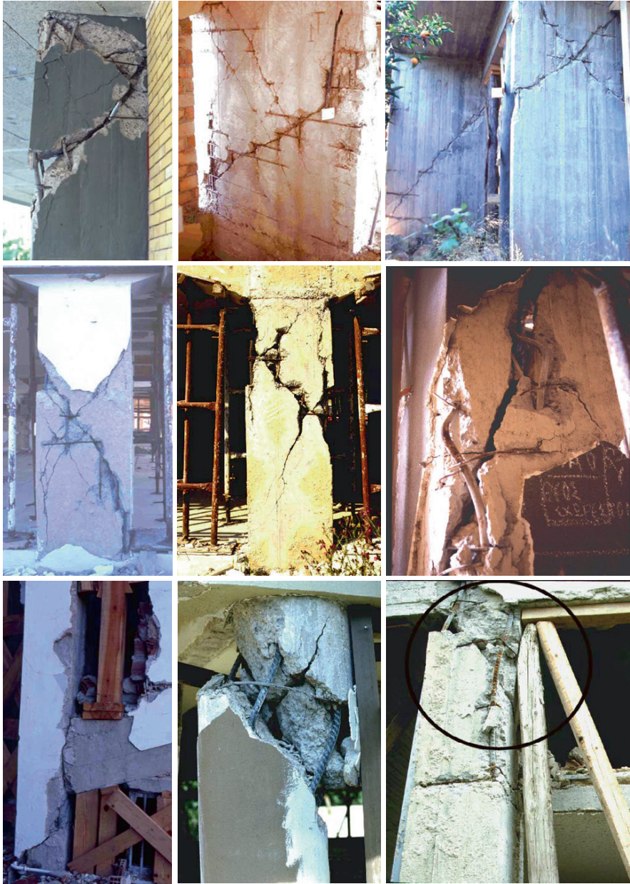
Plate 9 Shear failures of columns or walls (See also Figure 3.35 on page 252)
