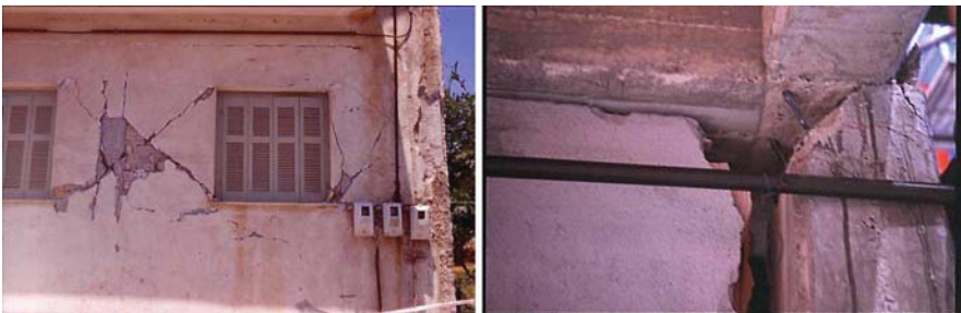
Fig. 2.11 Examples of shear failure of weak columns interacting with strong infills. (See also Colour Plate 2 on page 771)
