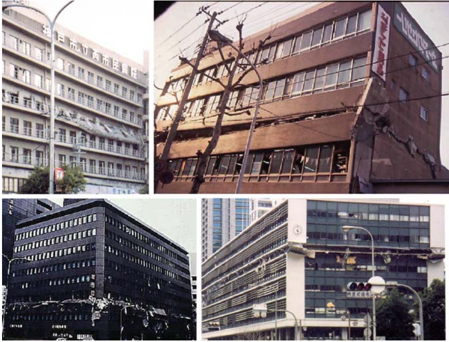
Fig. 2.4 Middle-storey collapses due to abrupt changes in stiffness or resistance of vertical elements (Kobe 1995)
