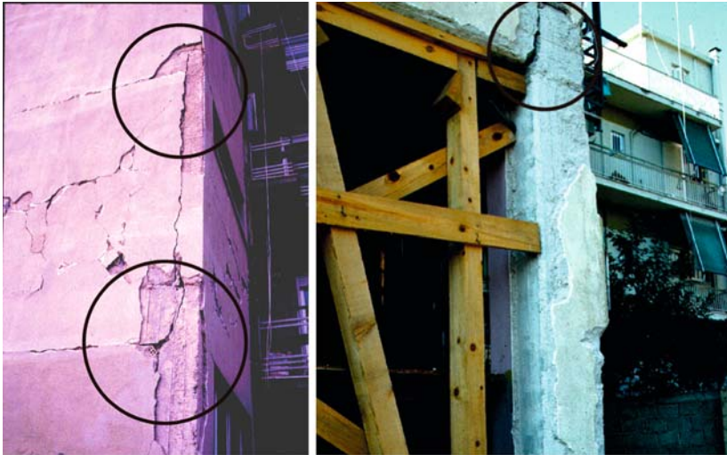
Fig. 3.29 Pull-out of beam bars from short anchorage in corner joint has produced fixed-end rotation during the response and wide residual cracks (See also Colour Plate 8 on page 722)
