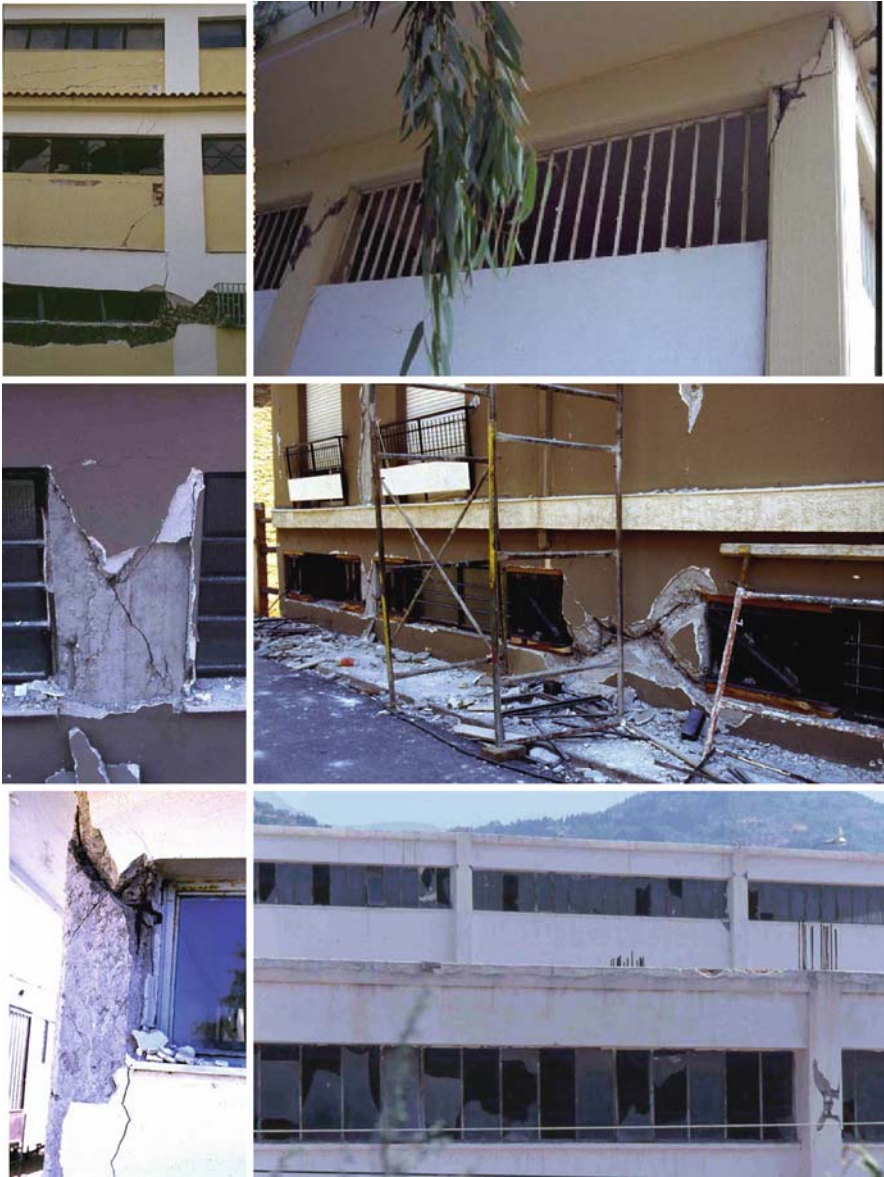
Fig. 2.12 Examples of captive column failures. (See also Colour Plate 3 on page 718)
