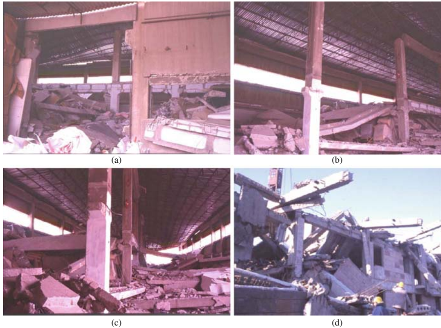
Fig. 2.7 Collapse of precast concrete buildings: (a)–(c) in Athens 1999; (d) in Spitak (Armenia) 1988
