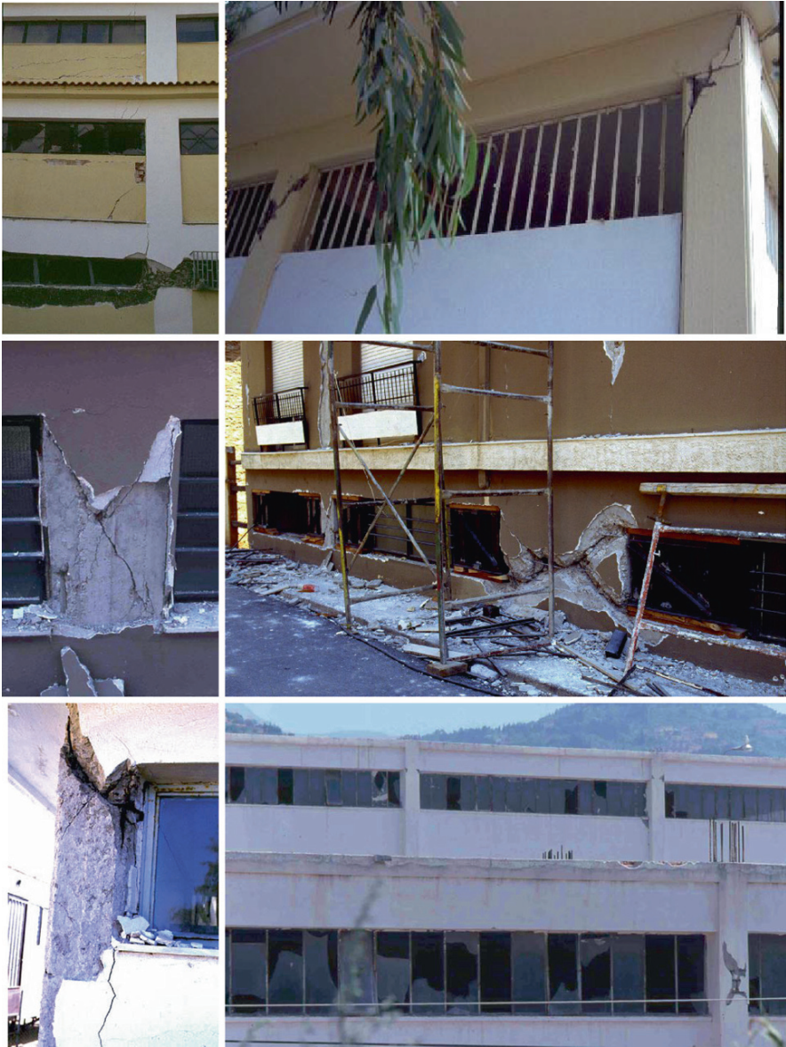
Plate 3 Examples of captive column failures. (See also Figure 2.12 on page 81)
