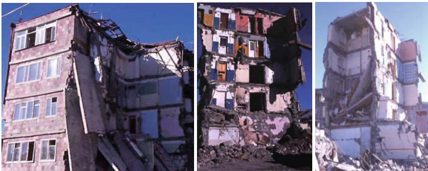
Fig. 2.6 Collapse of buildings with precast floors inadequately connected to the walls (Spitak, Armenia, 1988)
