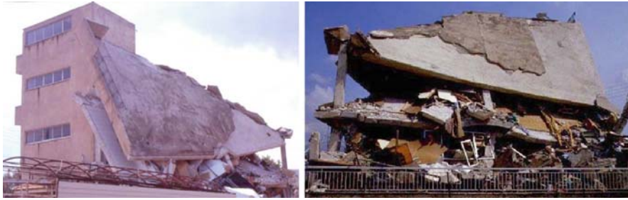
Fig. 2.1 Collapse of a building due to torsional response about a stiff shaft at the corner, Athens (1999) earthquake
