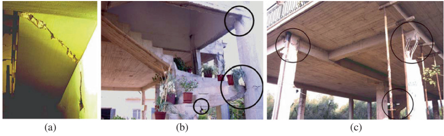
Plate 4 (a) Stair flight failing in shear as an inclined wall element in its strong direction; (b) corner stair in an open ground floor causes damage to the column it is connected to at mid-storey; and (c) columns at the diagonally opposite corner of the building failed during torsional response due to the stair in (b) – shown near bottom right at the back. (See also Figure 2.13 on page 82)
