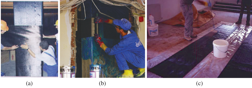
Plate 15 Hand lay-up of FRPs in situ: (a), (b) dry fabric impregnated in place (courtesy A. Ilki); (c) impregnation of the fabric right before placing (See also Figure 6.3 on page 654)
