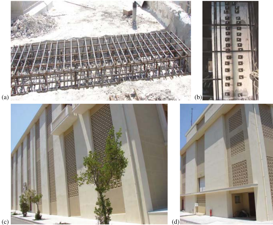
Fig. 6.15 Features of the retrofitting of the theatre building: (a) RC belt straddling joint at roof level; (b) steel rods connecting interior walls across the joint; (c) long side of the building with finished wall jackets; (d) new bay-long walls at the back
