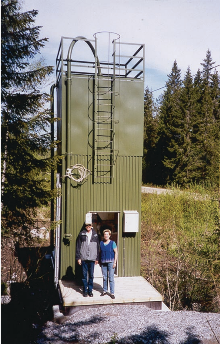
Fig. 22.2 Lime doser. In front Mats Näslund and Jorun Storeng from the Nordmaling Municipality administration. Photo by Johan Ahlström
