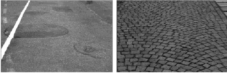
FIGURE 18.2. Typical defects of suburban and urban roads, relevant to vehicle comfort; at left a patched tarmac; at right a stone block pavement.
