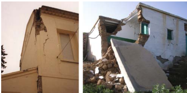
Fig. 9 Moderate and advanced corner damage to brick and adobe construction in Murcia and Al-Hoceima. (1999 and 2005 earthquakes)
