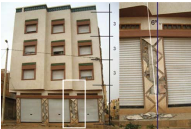
Fig. 12 Soft story damage with severely deformed ground floor and intact upper floors in Imzouren. (2004 Al-Hoceima earthquake)
