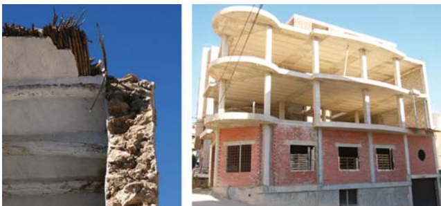
Fig. 2 Traditional fieldstone construction exposed in a damaged building and a typical contemporary RC frame construction for housing in Spain
