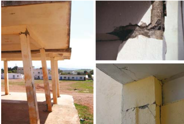
Fig. 11 Left : Severe damage to a RC portal frame in Imzouren during the 2004 Al-Hoceima earthquake. (grade 4) Top : Moderate fragile damage to a column and beam connection in Adra during the 1994 earthquake. (grade 3) Bottom : Moderate damage to a column and beam connection in Zarcilla during the 2005 earthquake. (grade 2)
