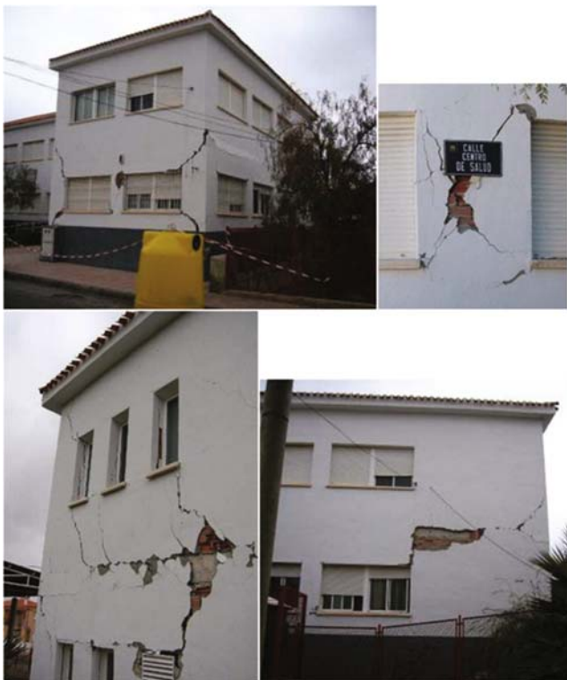
Fig. 19 Views of damage to external and internal infill panels in the Civic Centre of La Paca during the 2005 Lorca earthquake
