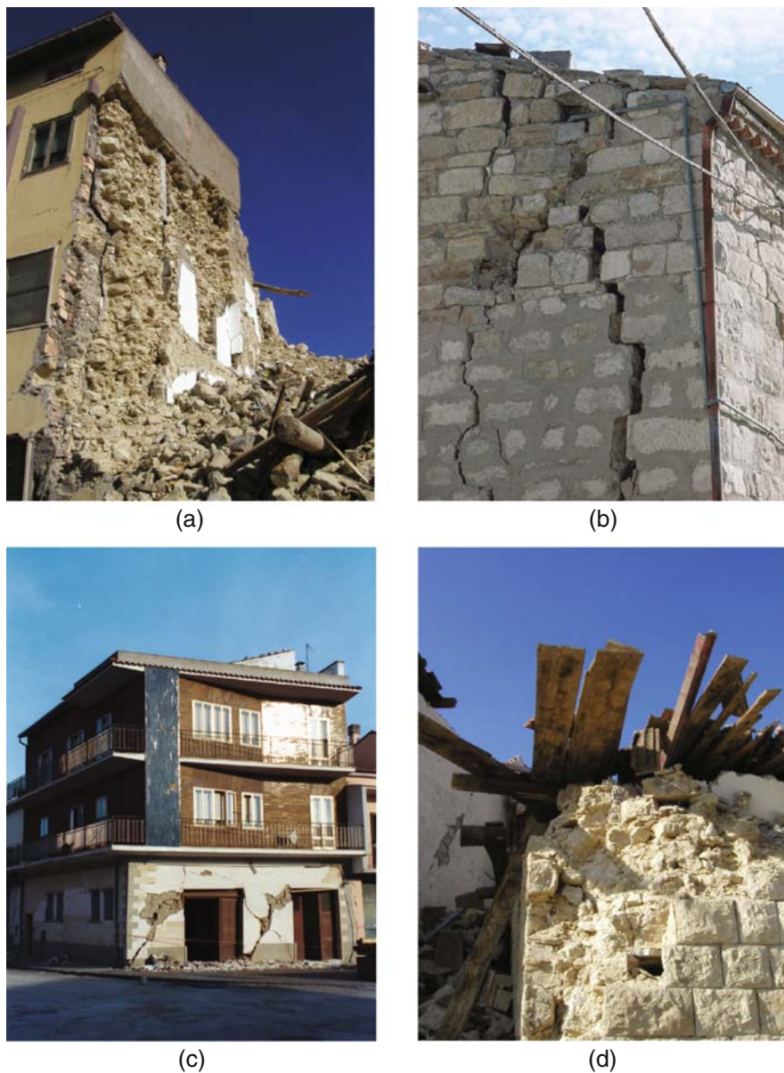
Fig. 2 Observed masonry buildings failure modes: (a) wall separation, (b) out of plane wall overturning, (c) in plane wall shear failure, (d) roof collapse
