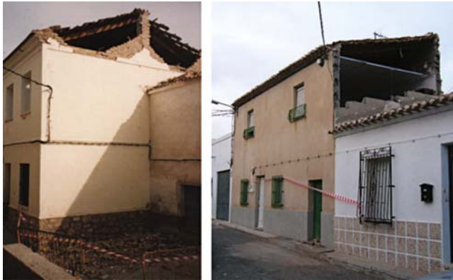
Fig. 8 Gable wall failure in brick and concrete block construction in Murcia, (1999 and 2005 earthquakes)
