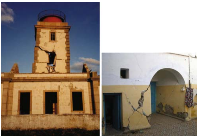
Fig. 6 Severe shear damage to the Punta Ribeirinha lighthouse in Faial Island (brick) and to a fieldstone masonry house in Tazaghine, Morocco. (1998 and 2004 earthquakes)
