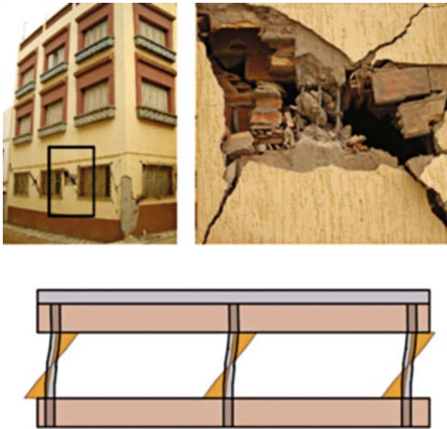
Fig. 15 Short column effect; damage to a column caused by interference of masonry panels in an apartment building in Imzuren. (2004 earthquake)
