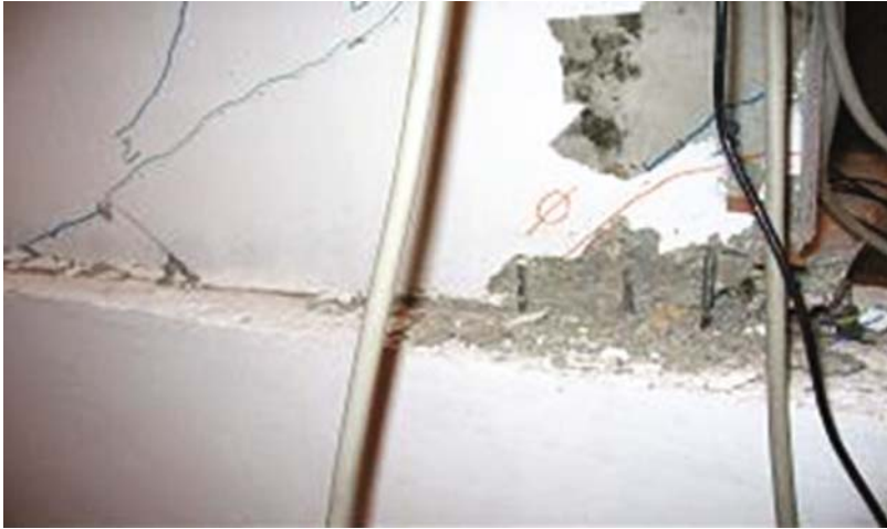
Fig. 18 Broken steel at the base of the wall X right for T6 motion
