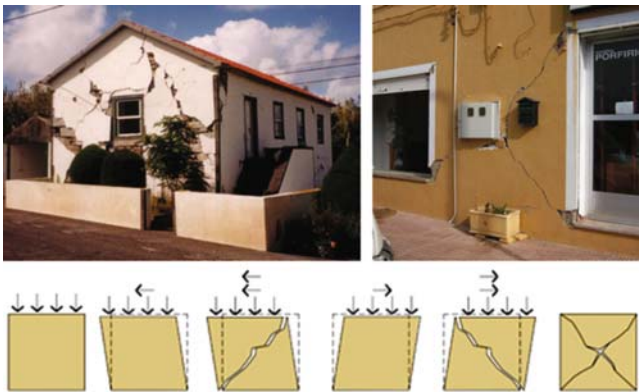
Fig. 5 Shear damage in fieldstone masonry construction in Cedros, Faial and Zarcilla, Murcia, (1998 and 2002 earthquakes) and model of X-crack generation in a masonry wall
