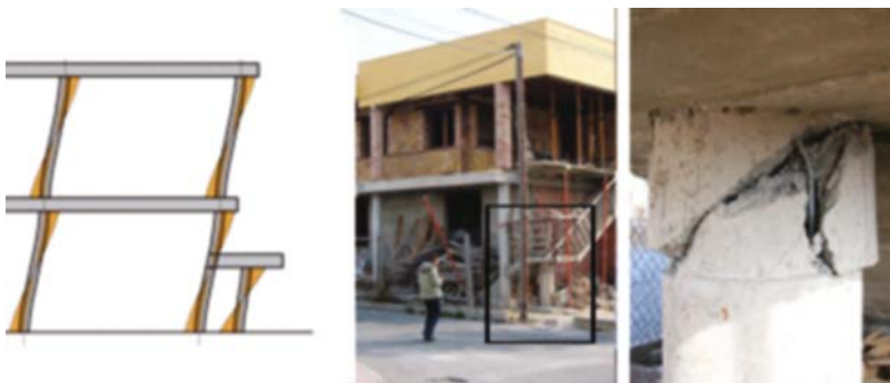
Fig. 16 Short column effect caused by geometric irregularities in Murcia. (2005 earthquake)
