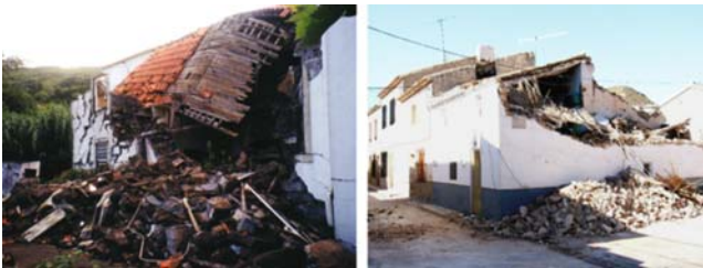
Fig. 10 Bearing wall collapse in Espalafatos, Faial Island and Murcia. (1998 and 2005 earthquakes)
