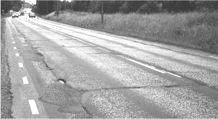
Fig. 13.38 An asphalt overlay over a concrete pavement showing severe reflection cracking. Reproduced by permission of MacPave Corporation
