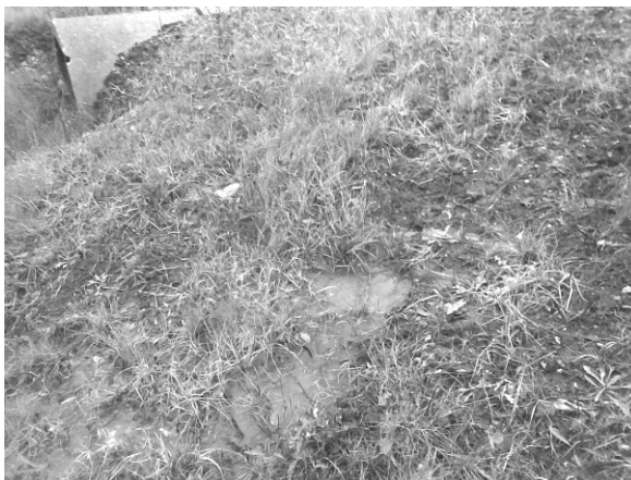
Fig. 13.45 Water exiting from an embankment slope where it has collected due to a culvert (in the background) acting as a barrier
