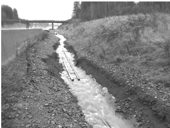
Fig. 13.34 Excessive run-off/seepage eroding the top of a drain following heavy rainfall
