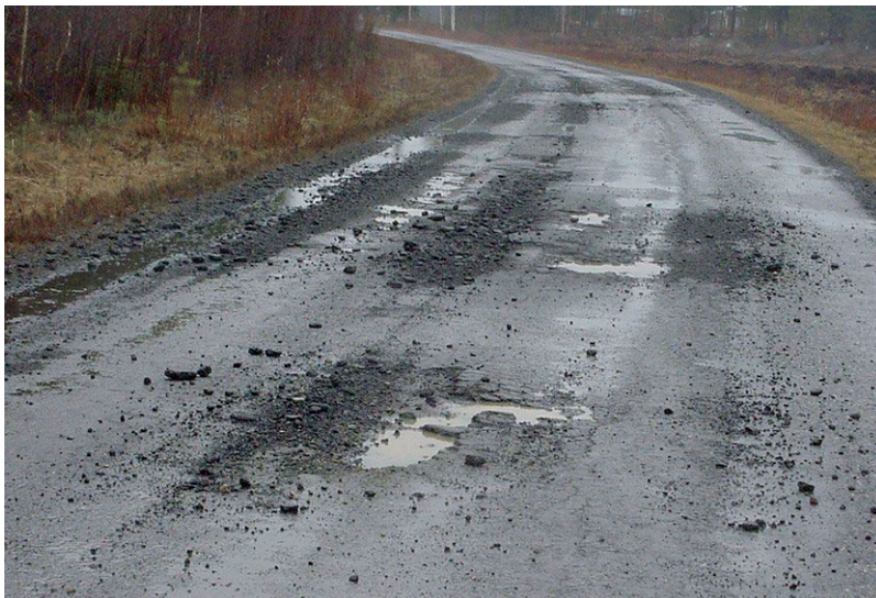
Fig. 1.9 Thin asphaltic surfacing of a road lifted by traffic-induced water pressure during spring-thaw in Northern-Karelia, Finland. Reproduced by permission of M. Leppänen
