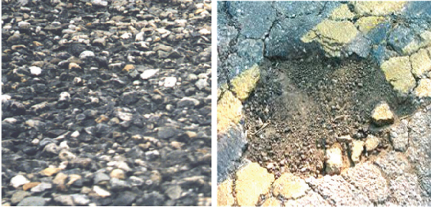
Fig. 5.4 Water-induced damage in asphaltic material (a) ravelling (b) potholing (de Bondt, 2005). Reproduced by permission of N. Kringos
