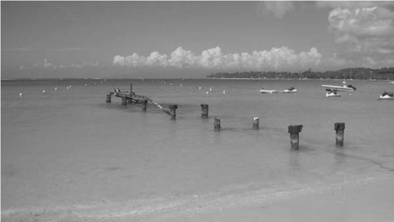
Fig. 15 Destroyed berth, Sainte-Anne
