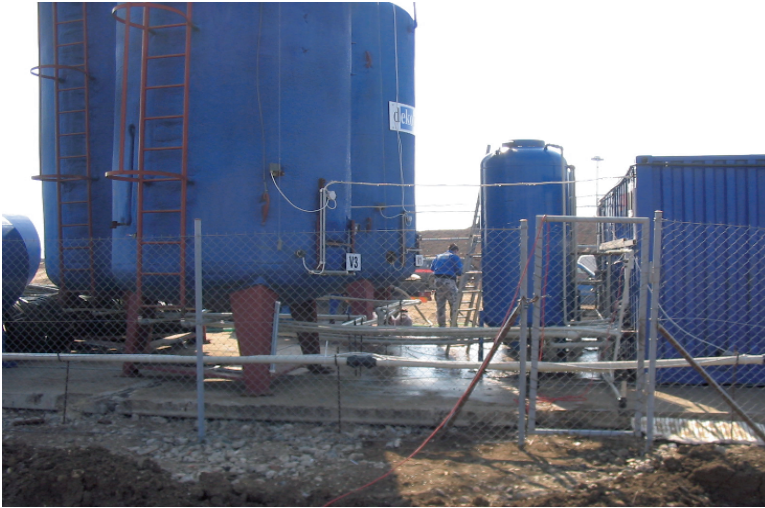
Figure 3. Biodegradation technological centre
