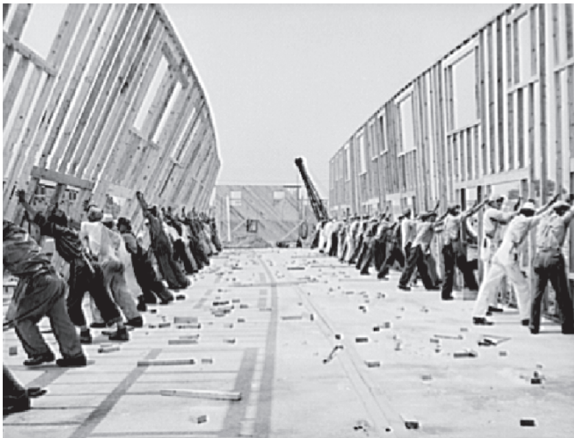
Fig. 2 Raising the framed walls of the balloon frame. 1941. (Alfred T. Palmer, photographer, 1941, Library of Congress, Prints & Photographs Division, FSA/OWI Collection, LC-USE6-D-000861.)
