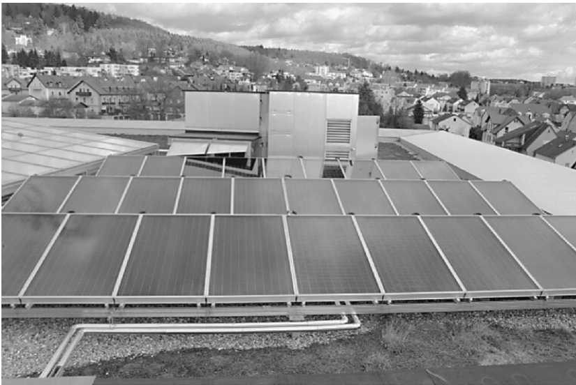
Figure 273. 70 m 2 collector array, in the background: casing of dehumidifier and regenerator
