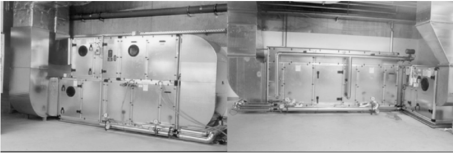
Figure 254. Heat exchanger and humidifier of the supply air and the indirect evaporative cooler of the exhaust air
