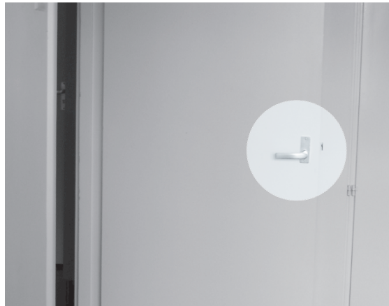
Figure 8. The user interface of a door is recognizable as a small protruding part.
