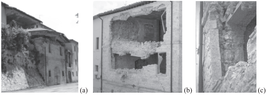
Figure 2. Brittle mechanisms detected in the upgraded buildings: (a) collapse of the upper floor of a building due to the substitution of the timber roof with a heavier r.c. and hollow tiles mixed one, supported by poor masonry walls; (b) rear of the same building where a large overturning of the façade occurred, due to the high percentage of openings, combined with the presence of a heavy r.c. floor supported by a single layer of the poorly connected double-layer masonry; (c) detail of the eccentric loading on the wall.
