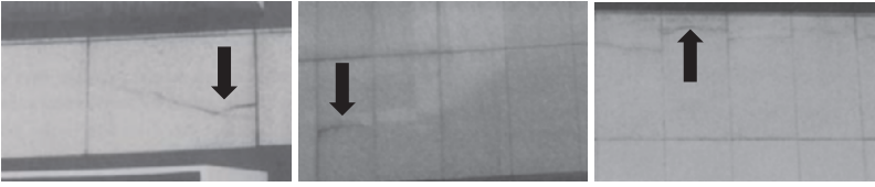
Figure 1. Typical cracking on granite cladding panels (Chew et al. 1 ).
